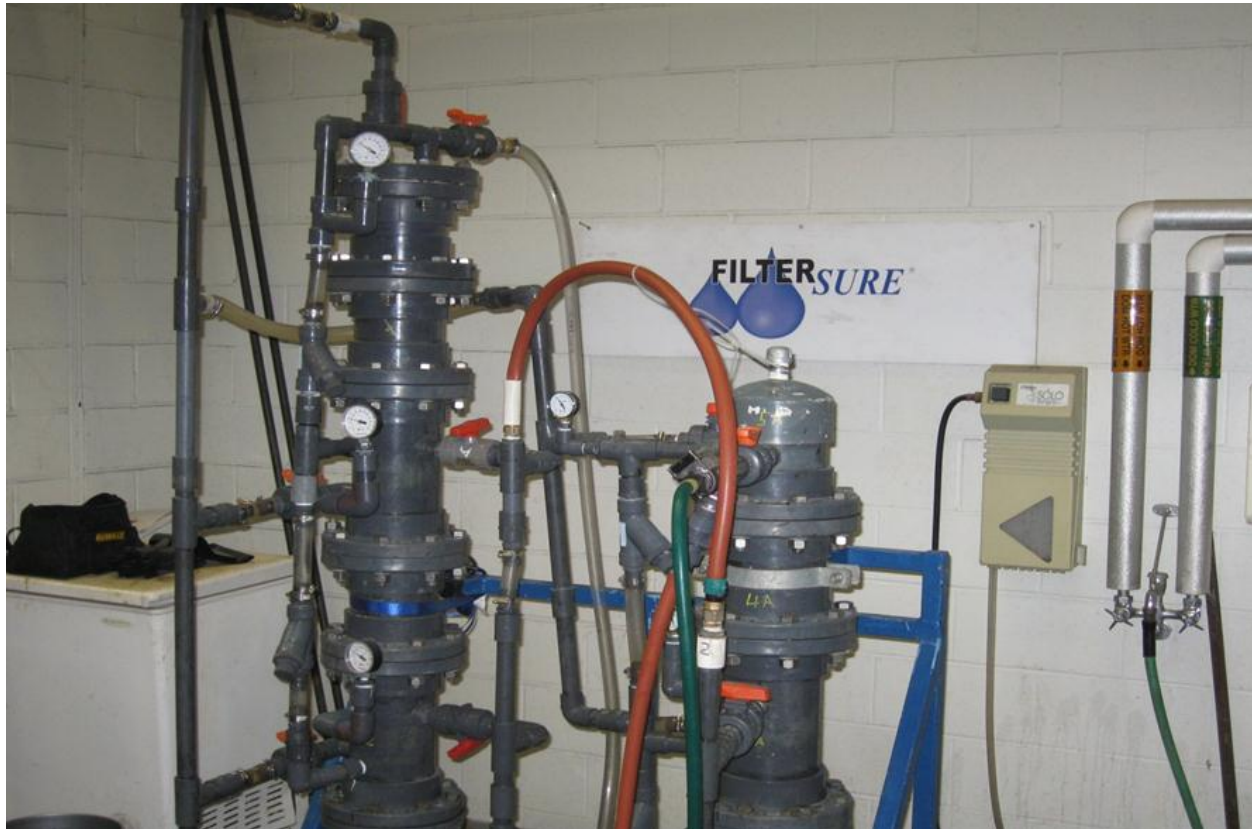
Figure 4: Media Testing of PDU for Treating Marcellus RFW
