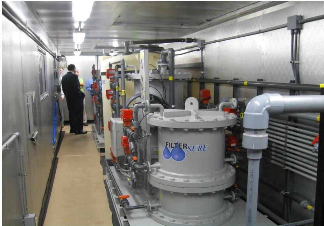
Figure 11: Completed Interior View of MTU
