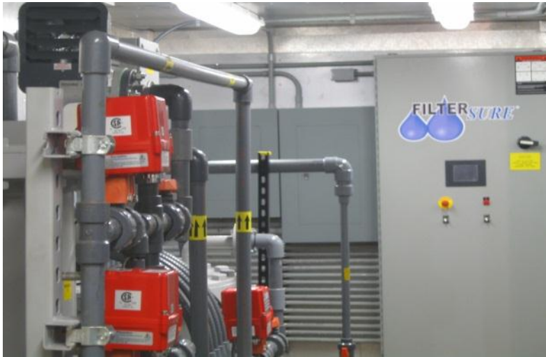
Figure 15: MTU Control Panel
