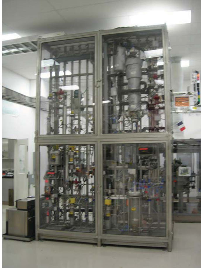
Figure 11 Bunsen section skid
