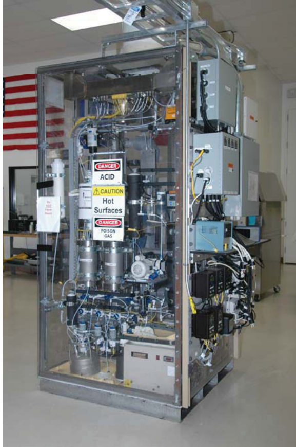
Figure 13 Sulfuric acid decomposition skid
