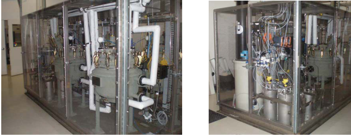
Figure 22 Interface Skid: I 2 /HI x tanks and Water/H 2 SO 4 tanks/Scrubber
