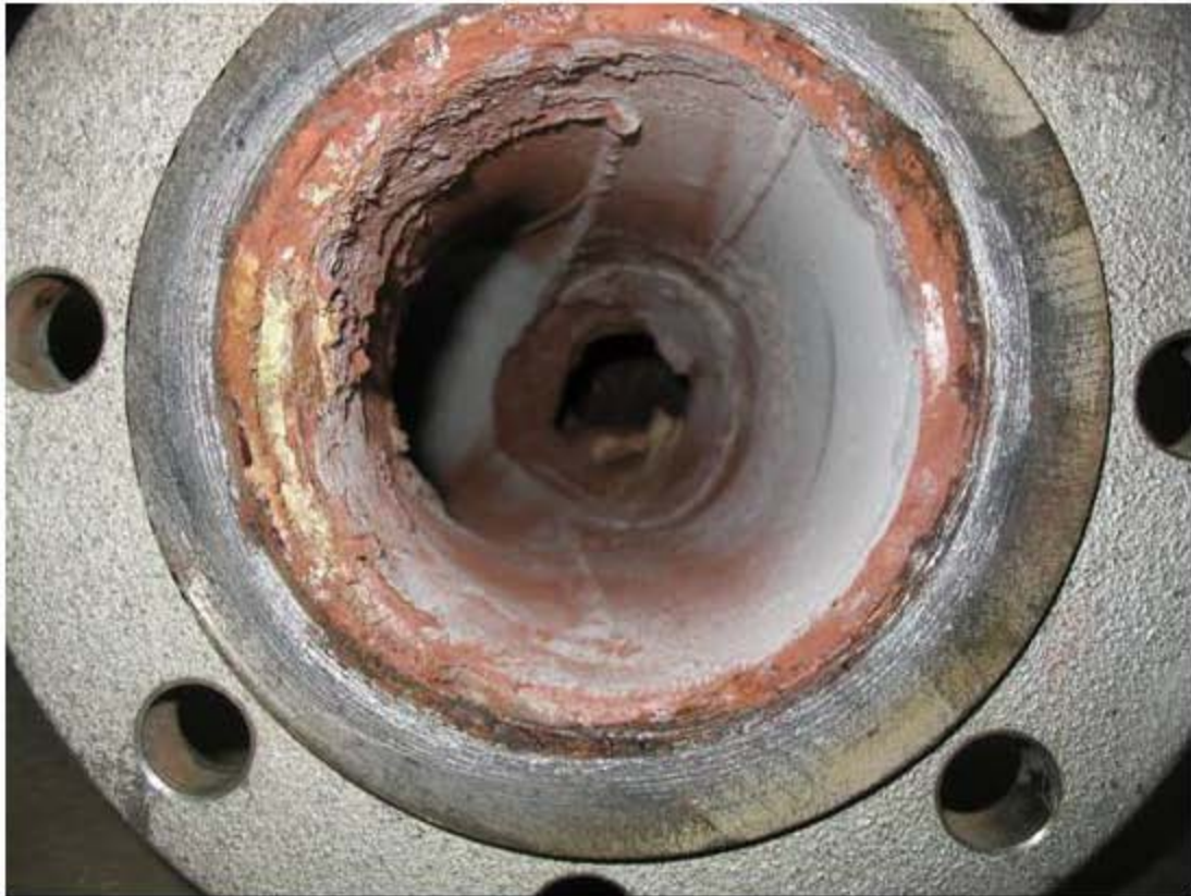
Figure 4.76. Outlet of transition line section in between the bellows and SBS inlet after HLW Turnover Test following the MACT tests [41].
