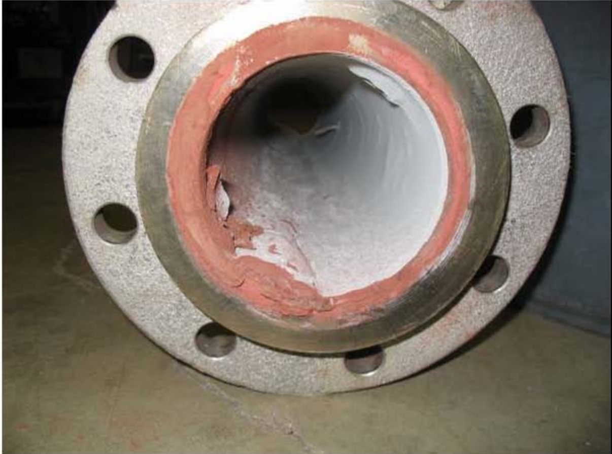
Figure 4.50. Transition line section #3 outlet after Configuration Test 10 [30].
