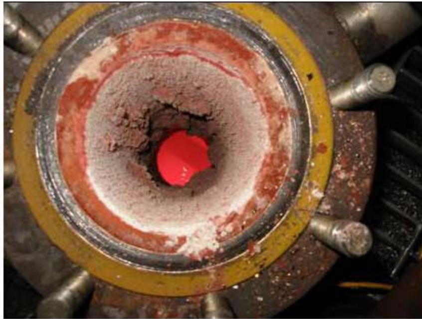
Figure 4.8. View of top of the installed film cooler after tests (pre-cleaning) with LAW Sub-Envelope Al simulants [14].
