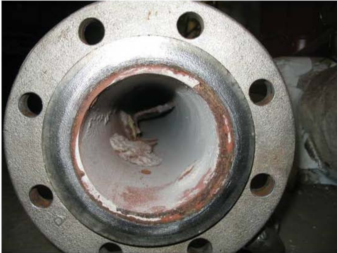
Figure 4.72. Transition line section #3 inlet after HLW Turnover Test following the MACT tests [41].
