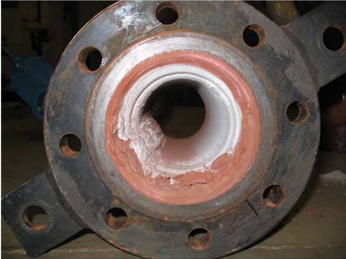
Figure 4.51. Transition line bellows inlet after Configuration Test 10 [30].
