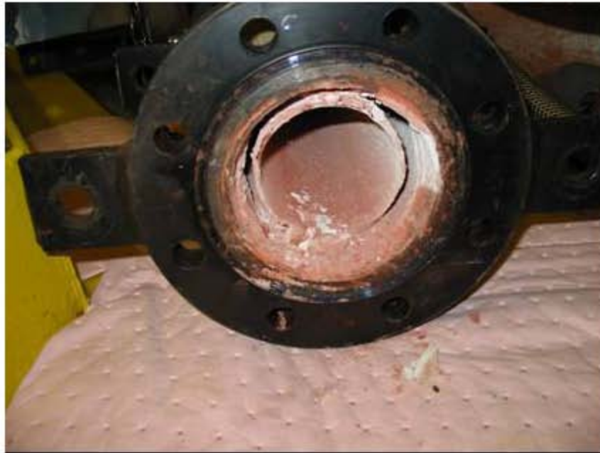
Figure 4.25. View of flexible bellows (pre-cleaning) during tests with LAW Sub-Envelope A1 simulants [14].
