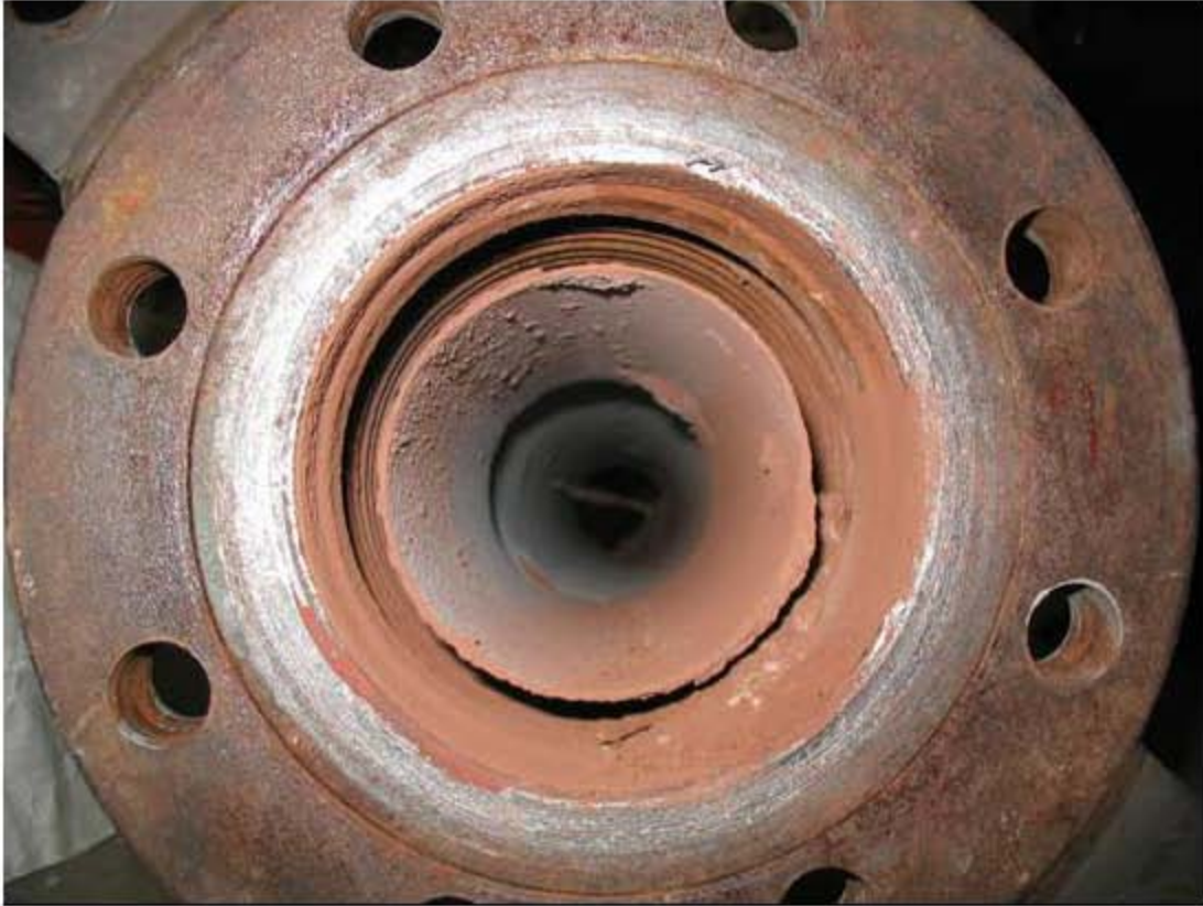
Figure 4.74. Transition line bellows outlet after HLW Turnover Test following the MACT tests [41].
