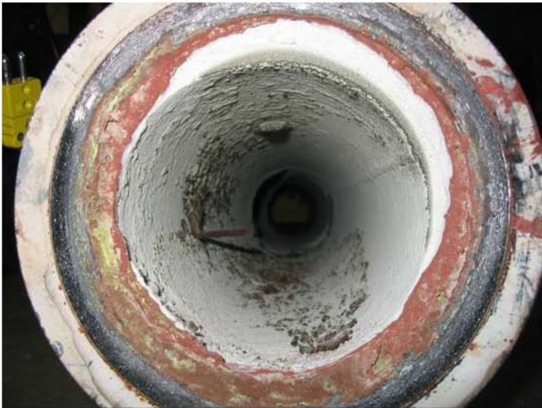
Figure 4.69. Transition line section #1 inlet after HLW Turnover Test following the MACT tests [41].
