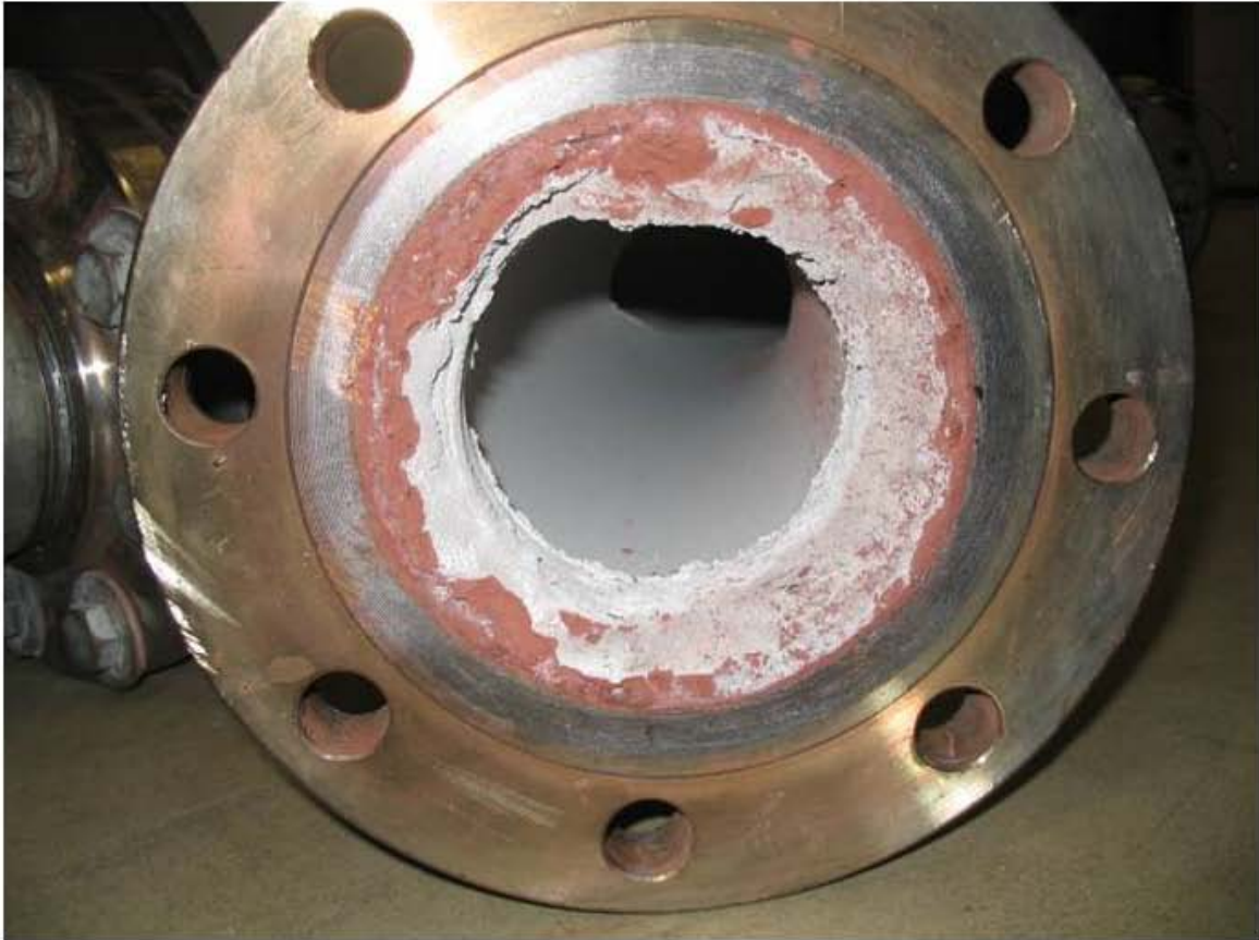
Figure 4.47. Transition line section #1 outlet after Configuration Test 10 [30].
