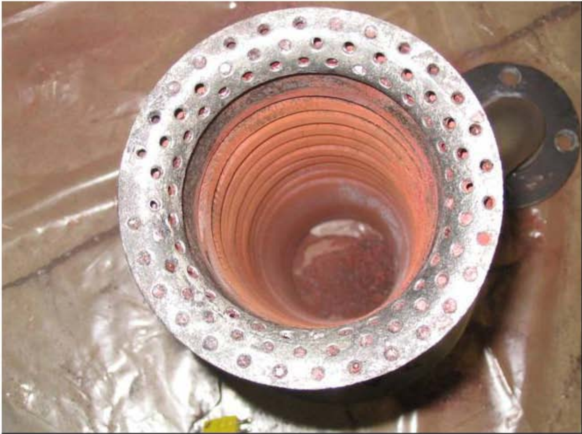
Figure 4.54. Film cooler inlet (post-cleaning) after Configuration Test 10 [30].
