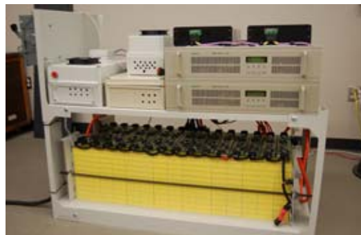
Figure 61. Greensmith Distributed Energy Storage System (DESS)
