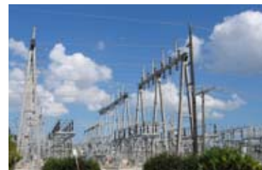
Figure 101. Flagami substation, side view (source: Meeker)
