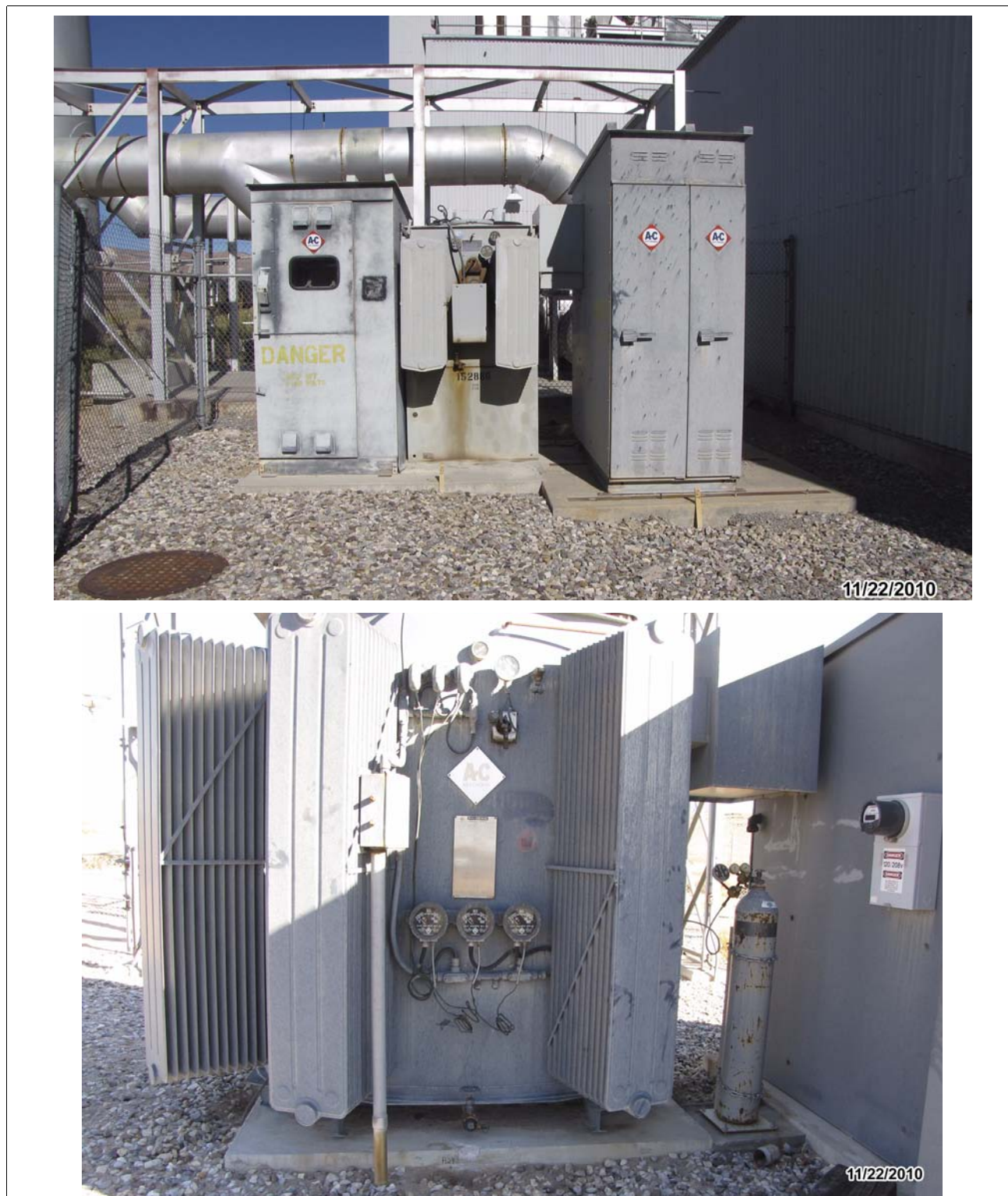
Figure 2-9 Southwest Electrical Substation (top) and Southeast Electrical Substation (bottom)
