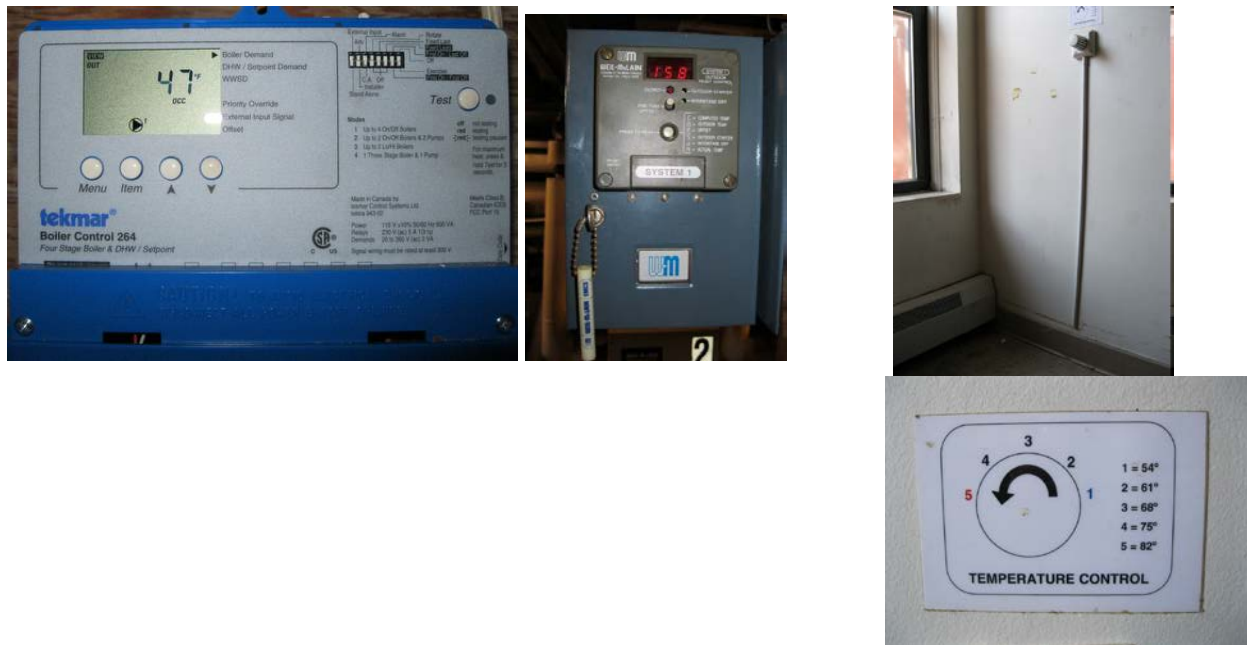
Figure 2. Existing boiler controllers (left and center) and local radiator controller (right)
