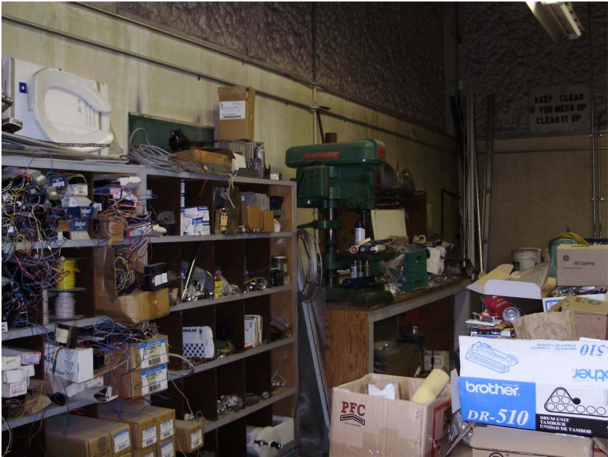
Previous central plant interior
