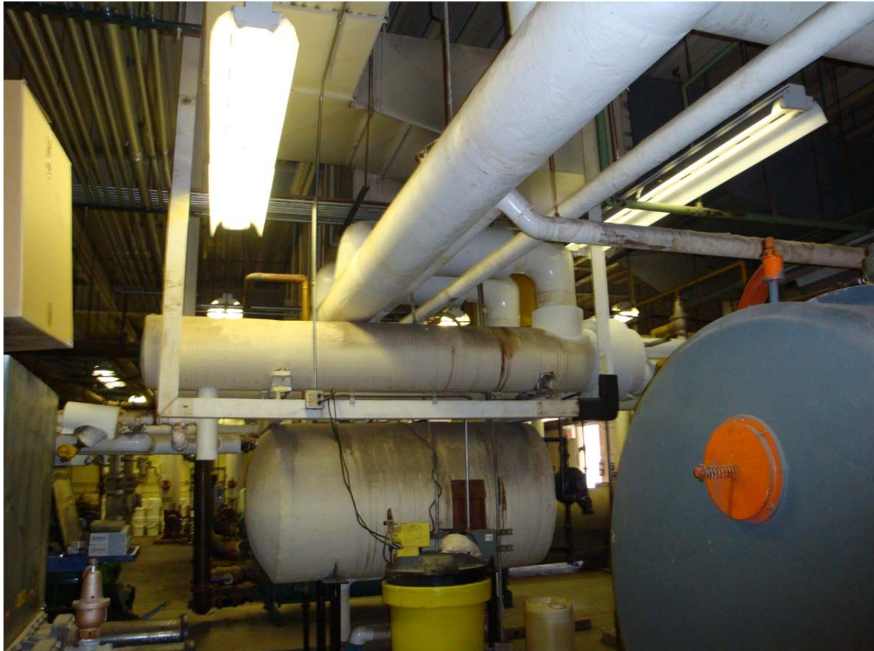
Previous boiler and hot water storage
