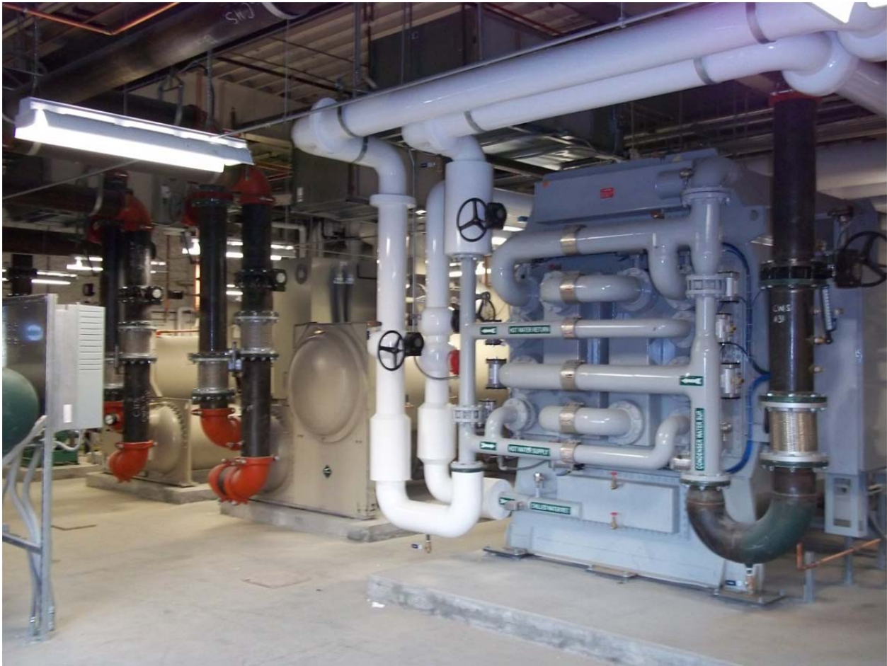
New adsorption chiller (on right) and new chillers (frictionless magnetic bearings)
