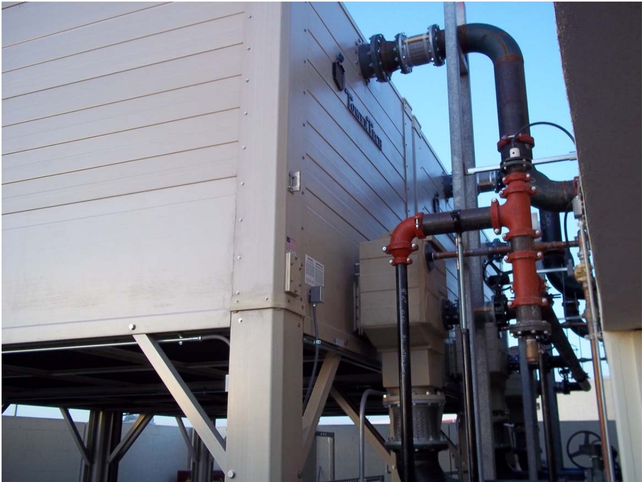
New cooling tower
