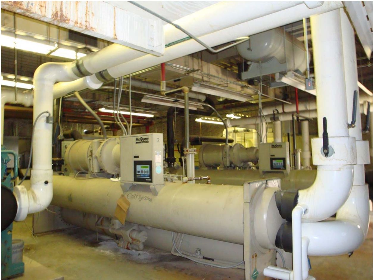
Previous (McQuay) chiller (same as last image)
