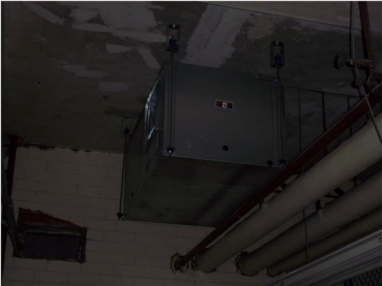
New water source heat pump
