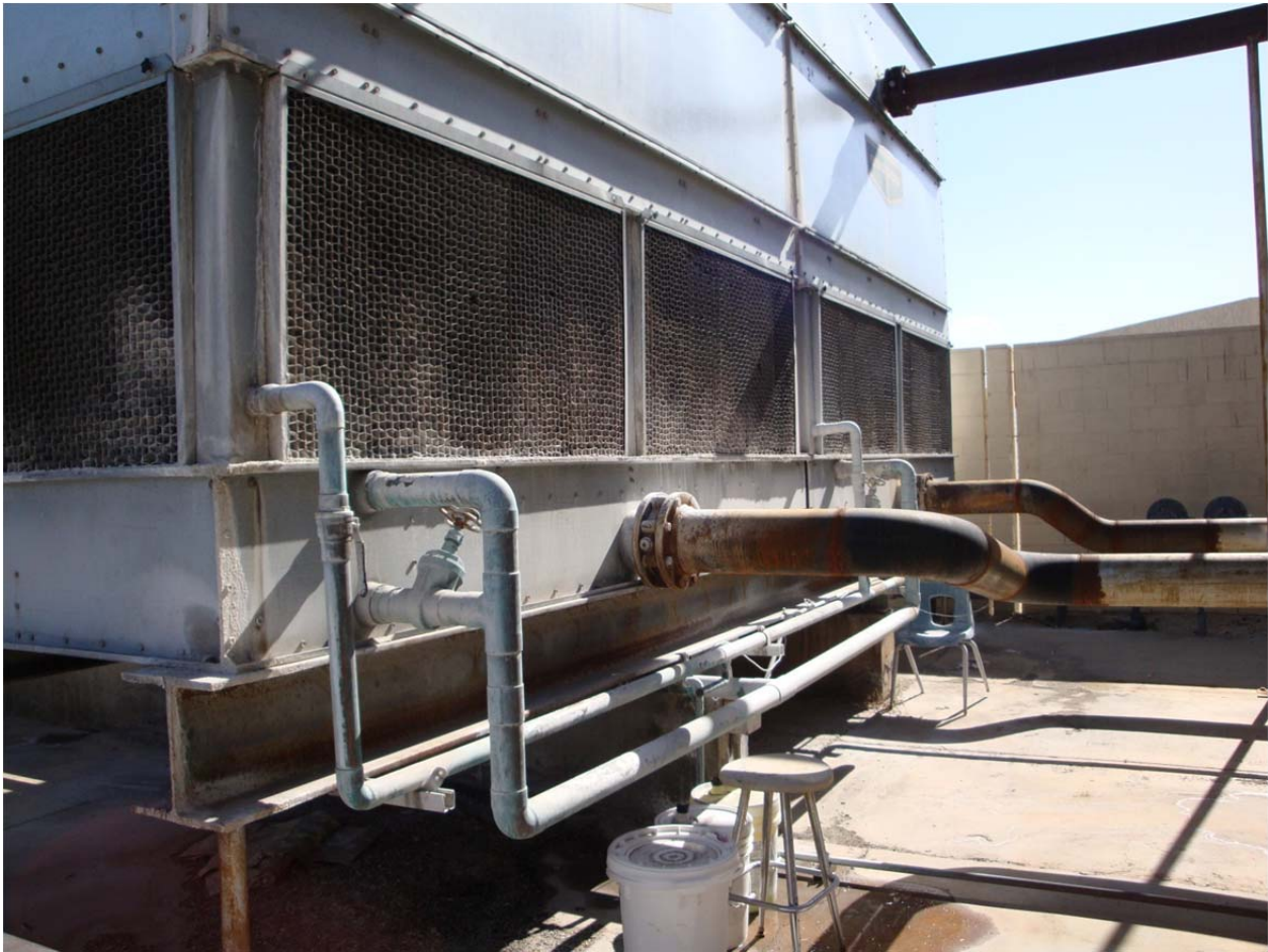
Previous cooling tower
