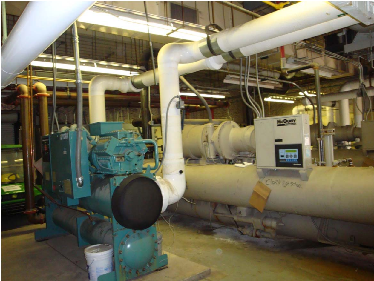
Previous (McQuay) chiller
