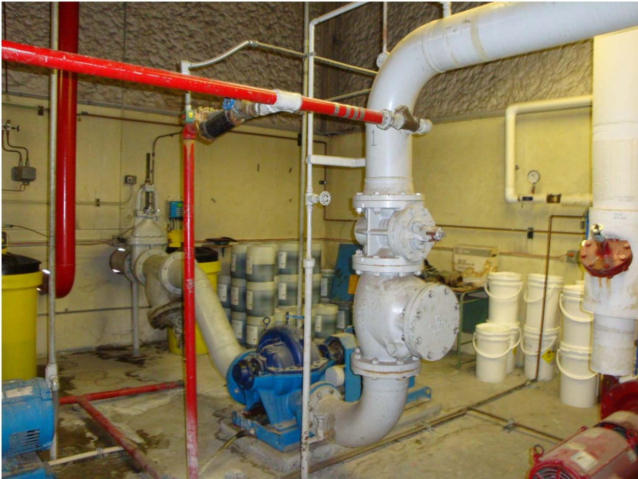
Previous condenser water pump
