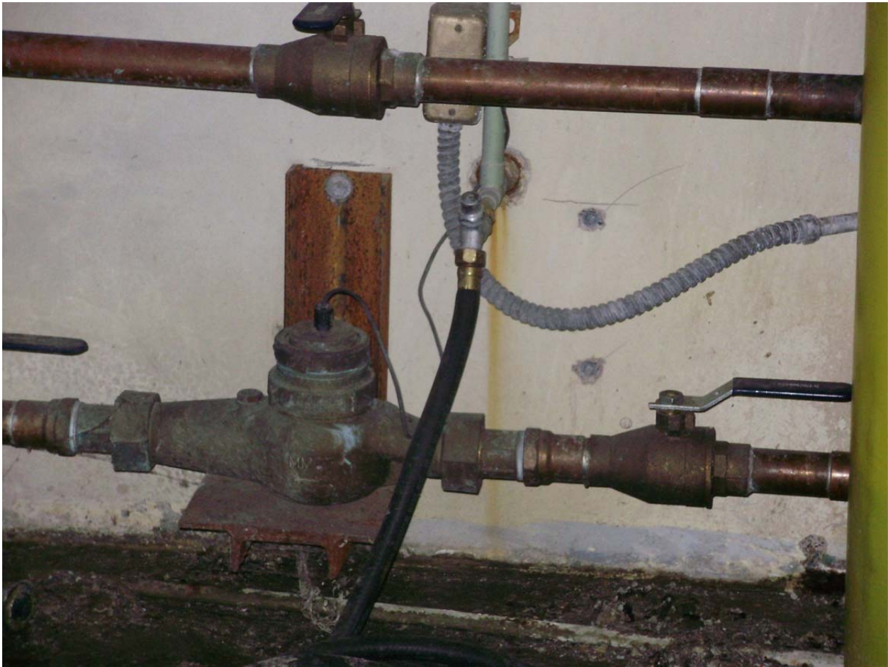
Previous central plant interior
