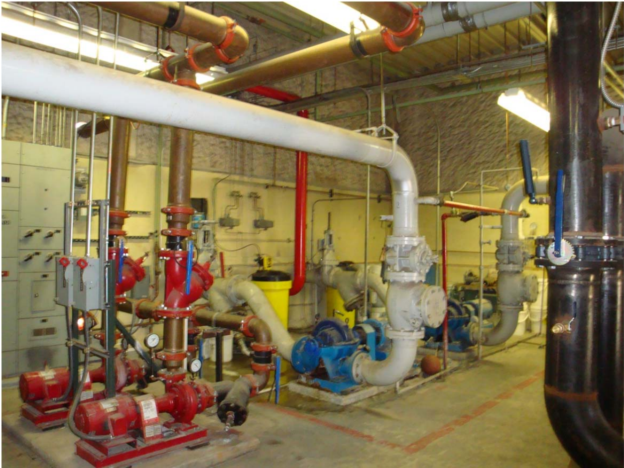
Previous hot water and chilled water pumps
