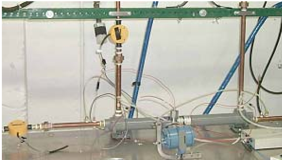
Figure 6.12. Close-up view of the laboratory heat exchanger.
