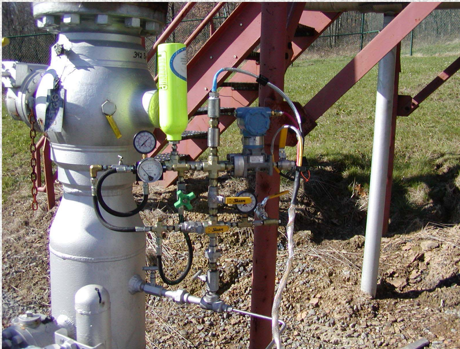
Figure 5 - Second generation Portable Acoustic Monitoring Package (PAMP) weighing only 36 pounds mounted on a transmission line from Dominion Transmission Inc.
