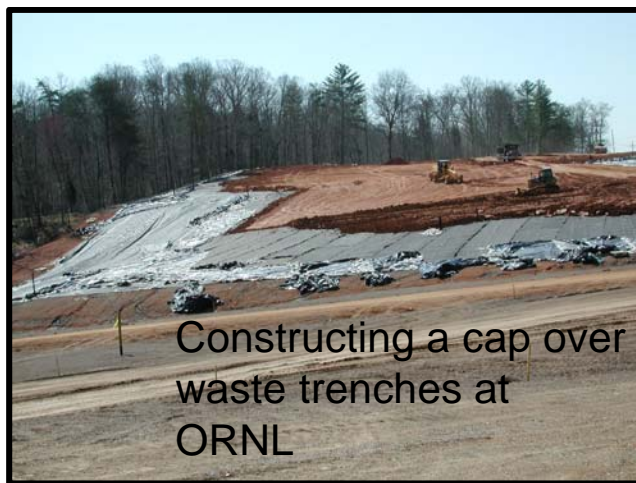
Figure 3: Recent capping activities on the Oak Ridge Reservation in an effort to impede infiltrating storm water from entering subsurface waste trenches.
