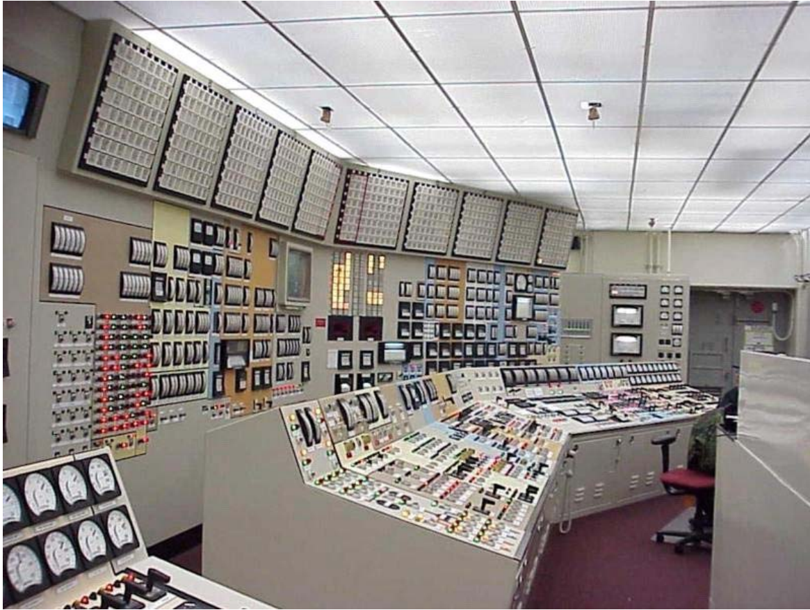
Figure 2-5 Photo of an Existing U.S. Nuclear Power Plant Control Room
