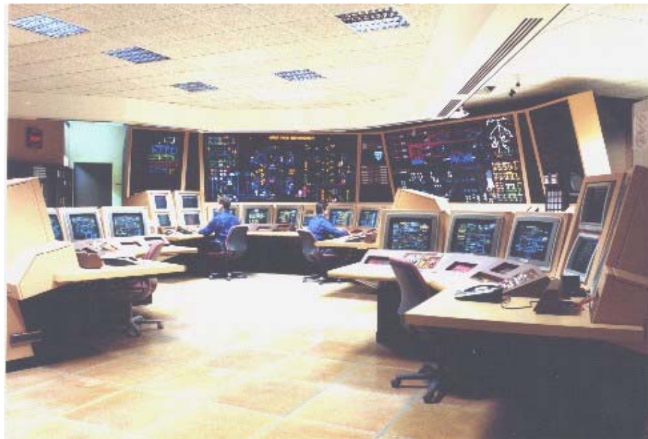
Figure 2-7 Photo of a Modern Control Room Built in France
