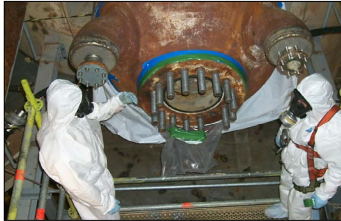
Picture 2: the steam generator during final rinsing and inspection
