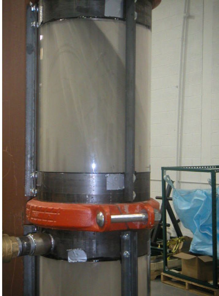
Figure 4. Test Section flowing Silicon and Air Offset elbows upstream used to induce swirl flow
