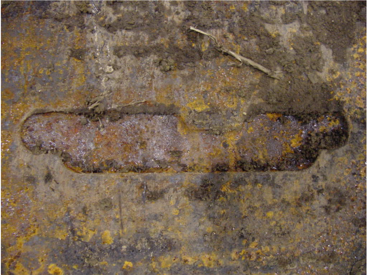
Figure 95 - Simulated Corrosion on Outside of Pipe After Internal Weld Deposition Repair
