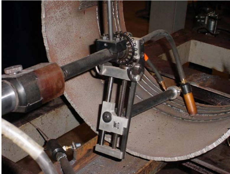
Figure 31 - Bortech Torch and Torch Height Control
