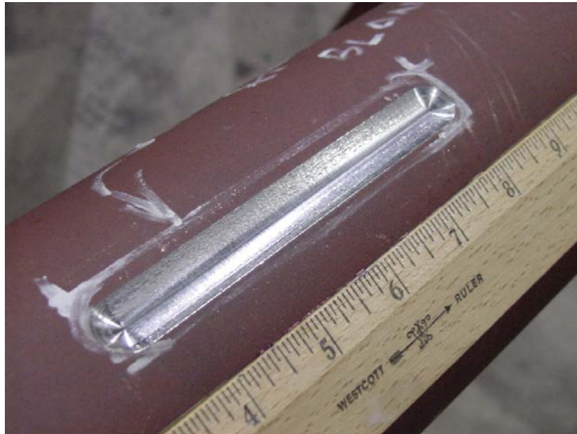
Figure 12 - Long, Shallow Simulated Corrosion Damage
