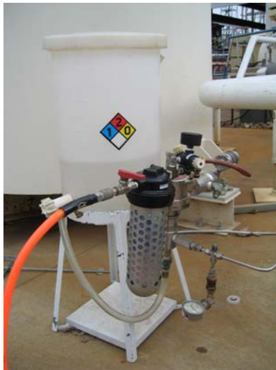
Fig 4.7 Foam Breaker Pump
