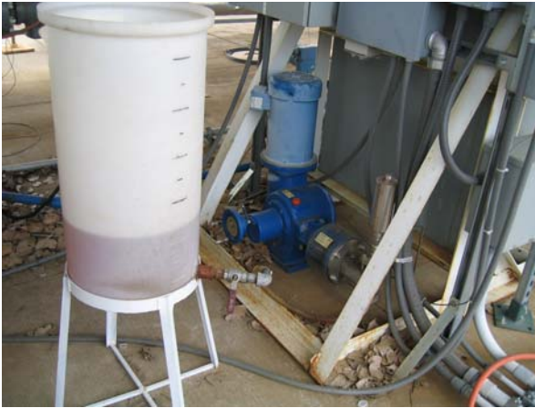
Fig 4.5 Surfactant Injection Metering Pump
