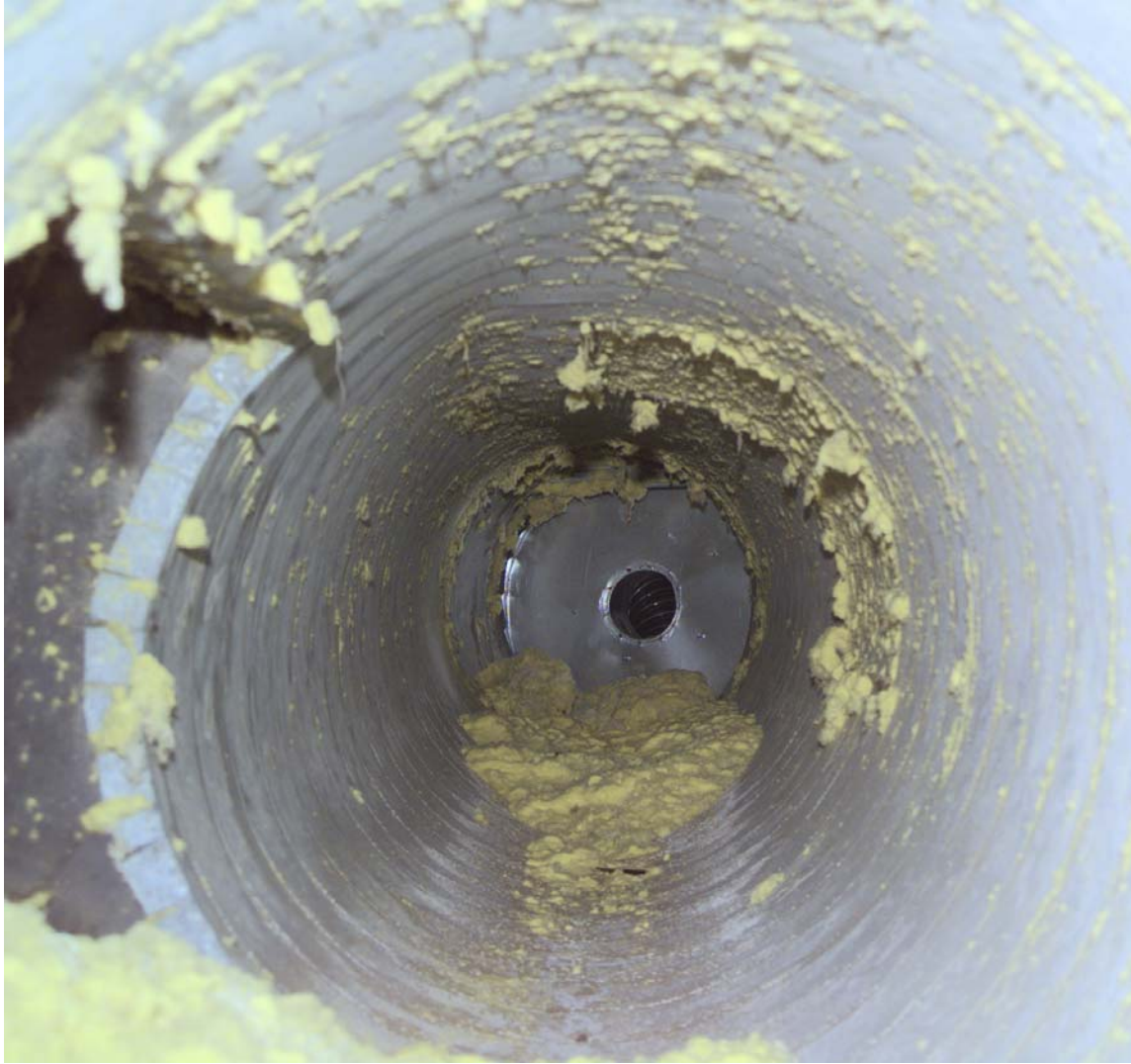
Figure 2. Excessive Lint in the CFA-617 ducting prevented the fogging from working effectively.
