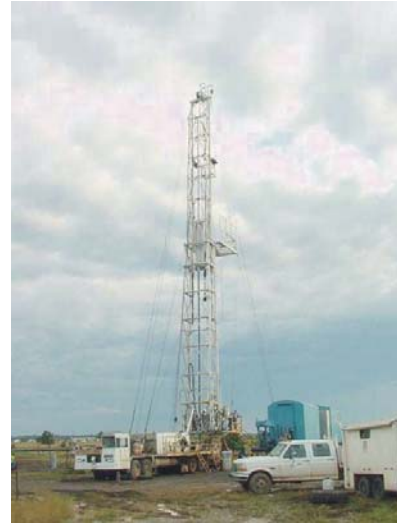
Well Site: French 4-4, Leflore County, OK 100 ft. High Drill Rig operated by Rambler Energy Services.
