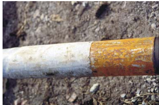
Condition of joint end after use a little rust on the steel end, but the composite has only a few scratches.
