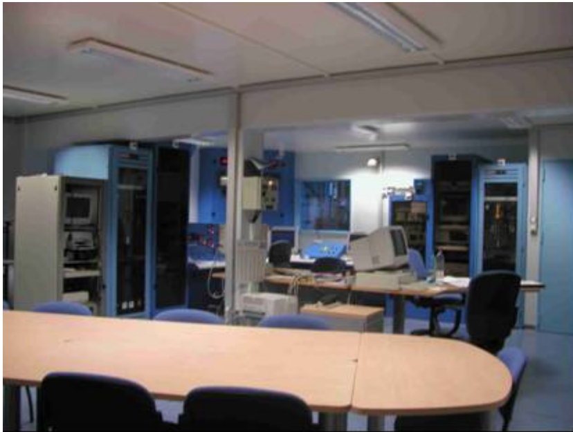
Figure 1: Photo of the new control room
