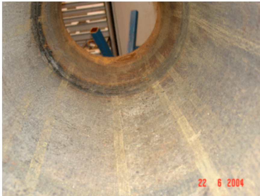
Figure 10. Cast Iron Pipe ID after Cleaning
