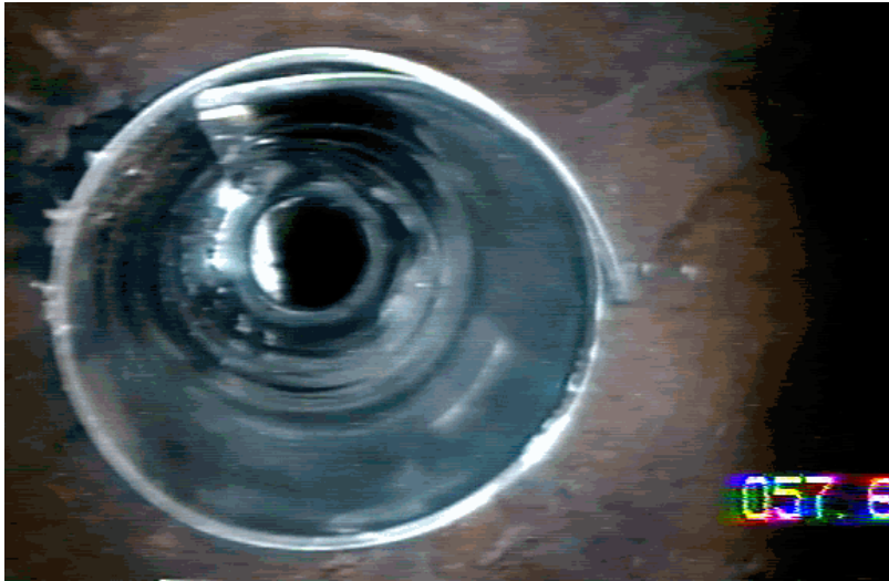
Figure 44. Partially Engaged Patch at 58.6 ft
