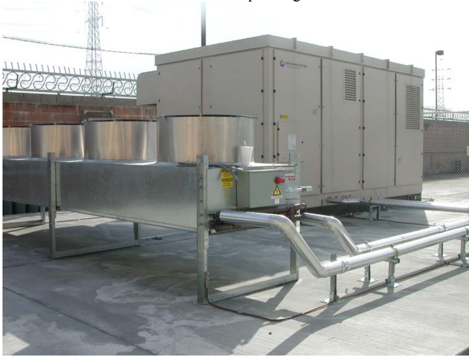
PC25C fuel cell power plant at the Main St. Facility in full load operation
