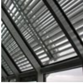
Automated tubular grid skylight controls daylight at Munich Airport.
