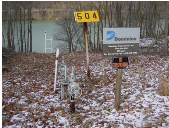
Figure 1 – Dominion line 323 near Morgantown, WV, the 1/2" NPT inspection ports can be seen located on either side of the shut-off valve.
