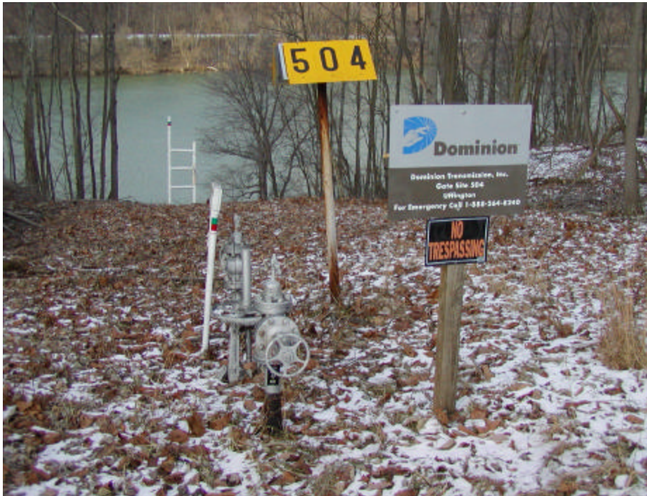
Figure 1: Dominion line 323 near Morgantown, WV, showing the ½" NPT inspection ports on either side of the shut-off valve.
