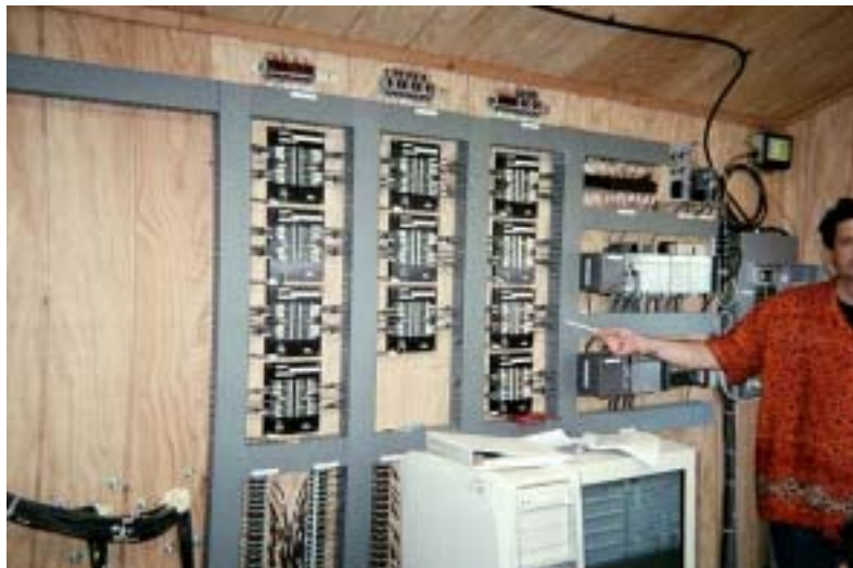
Image 7-1: Completed hardware installation
