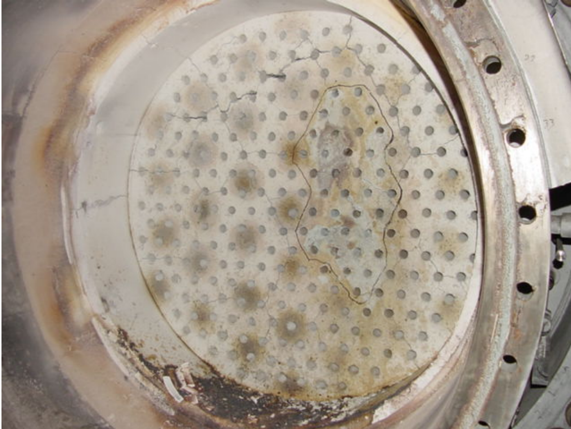
Figure 2 Picture of failed pulse combustor tube sheet.
