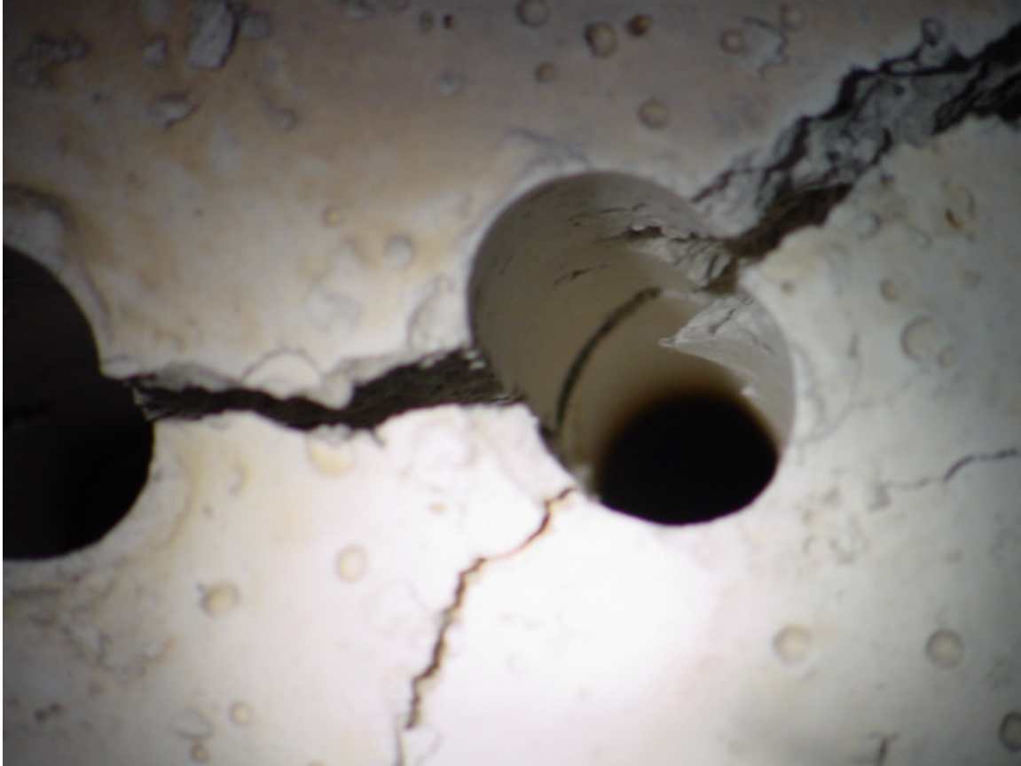
Figure 3 Enlargement showing critical delamination failure at 5-6" in depth and accompanying transverse cracking.
