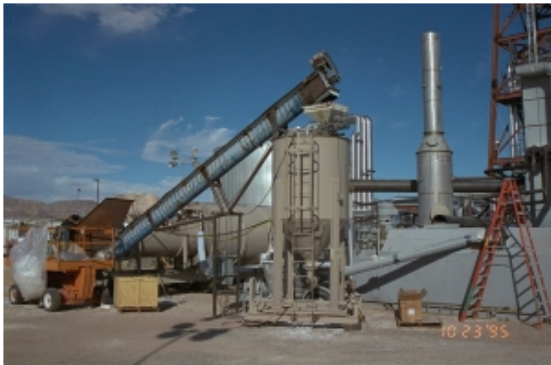
Figure L-4. Conveyor belt feeding crushed salt from the hammer mill into the salt hopper. The screw auger can be seen as the pipe feeding into the wall next to the ladder. The vent stack to dilute the NO x can be seen in the background.
