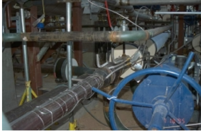
Figure Q-3. Multiple heat trace cables were applied to pipes that drained nightly to allow a two-hour heatup time the next morning. One or two spare cables were installed as well. A lesson learned was that heat trace must be installed uniformly (i.e. constant value of W/ft); otherwise, hot spots can occur that lead to pipe corrosion. A nonuniform section of heat trace is seen in this photo (see loop back). During the rework of the heat trace system in 1996, nonuniformities were eliminated.
