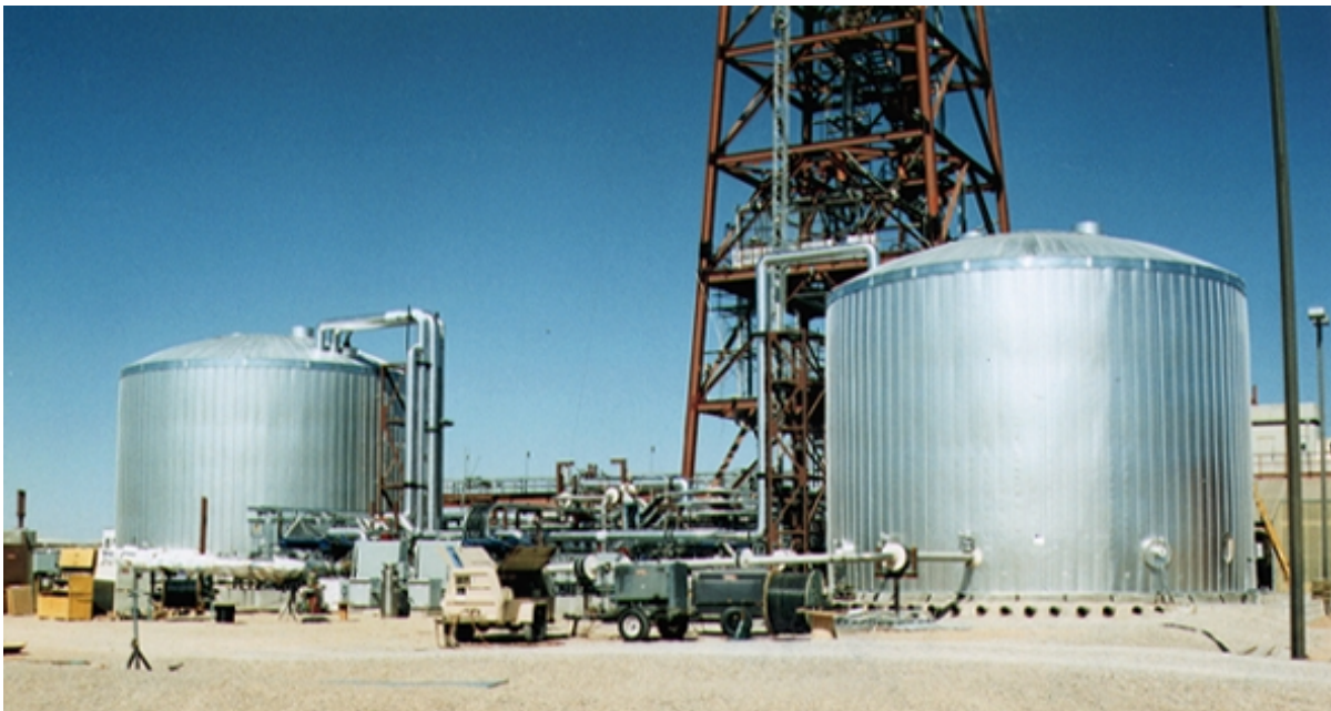
Figure 4-1. Cold (left) and hot (right) nitrate salt storage tanks.
