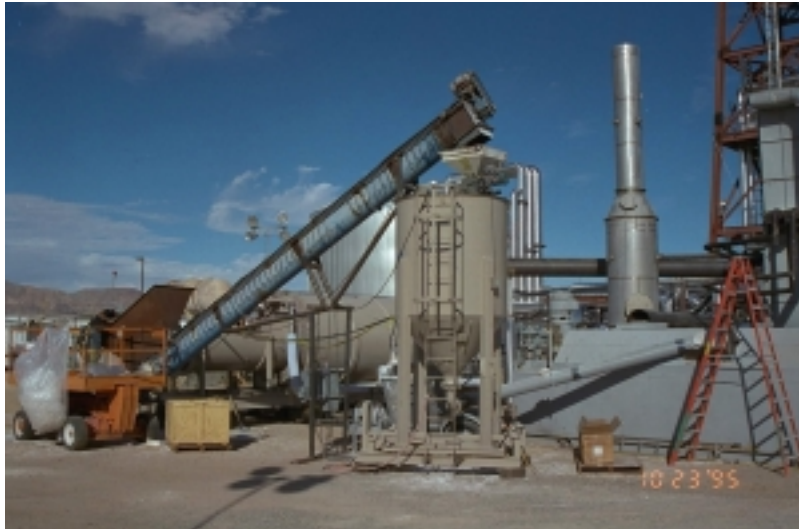
Figure 4-4. Conveyor belt feeding crushed salt from the hammer mill into the salt hopper. The screw auger can be seen as the pipe feeding into the wall next to the ladder.
