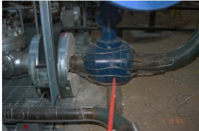
Figure Q-4. Valves can be kept warm overnight, independently of the surrounding pipe, if a separate heat trace circuit is applied to the valve. This reduces parasitics because the pipe heaters can be turned off at night. In this photo, the same heat trace circuit was applied to the valve and surrounding pipe. During the rework of the heat trace system in 1996, separate valve circuits were installed on valves 4 inches in diameter and bigger.
