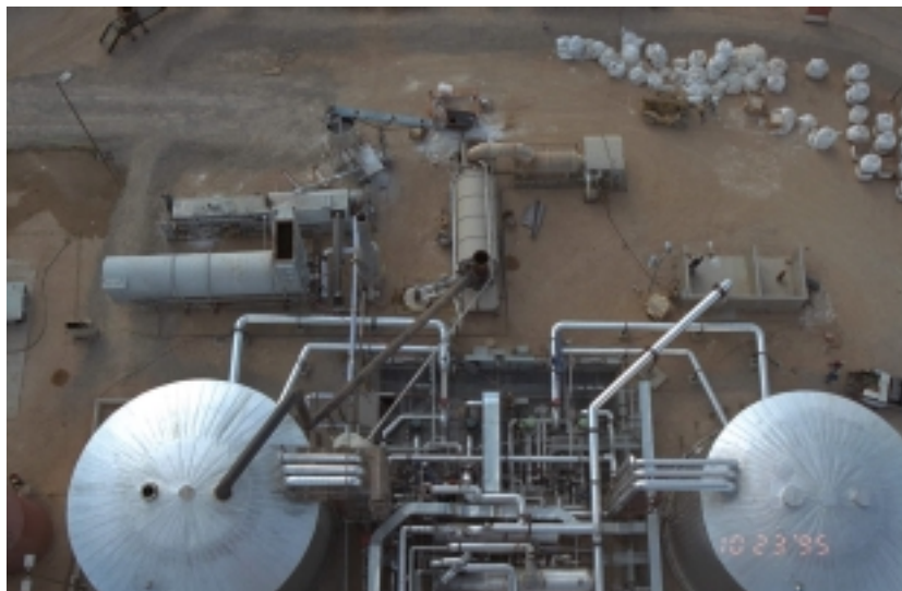
Figure L-5. Overhead view of the salt fill operation; the hot tank is on the left and the cold tank is on the right.
