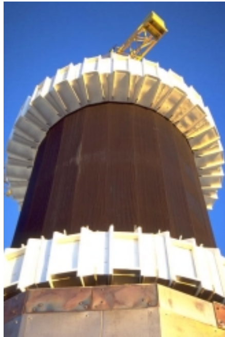
Figure 3-1. Close-up of Solar Two receiver.
