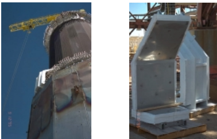
Figure Q-2. Ovens structures surround the receiver header pipes. Seals must be good for ovens to be effective. Sealing problems often made it difficult to heat up the ovens on the windward side of the receiver.
