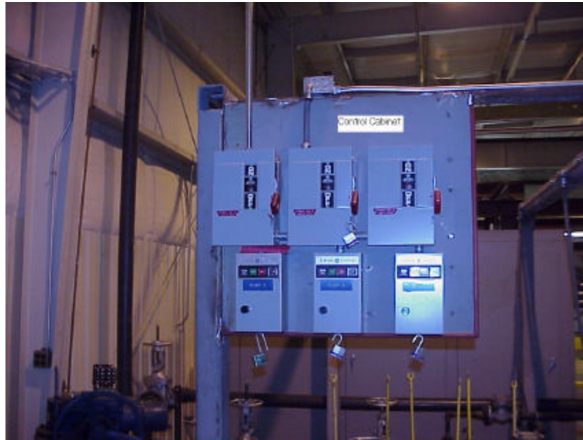
Figure A.4: Motor Control Panel Closed
