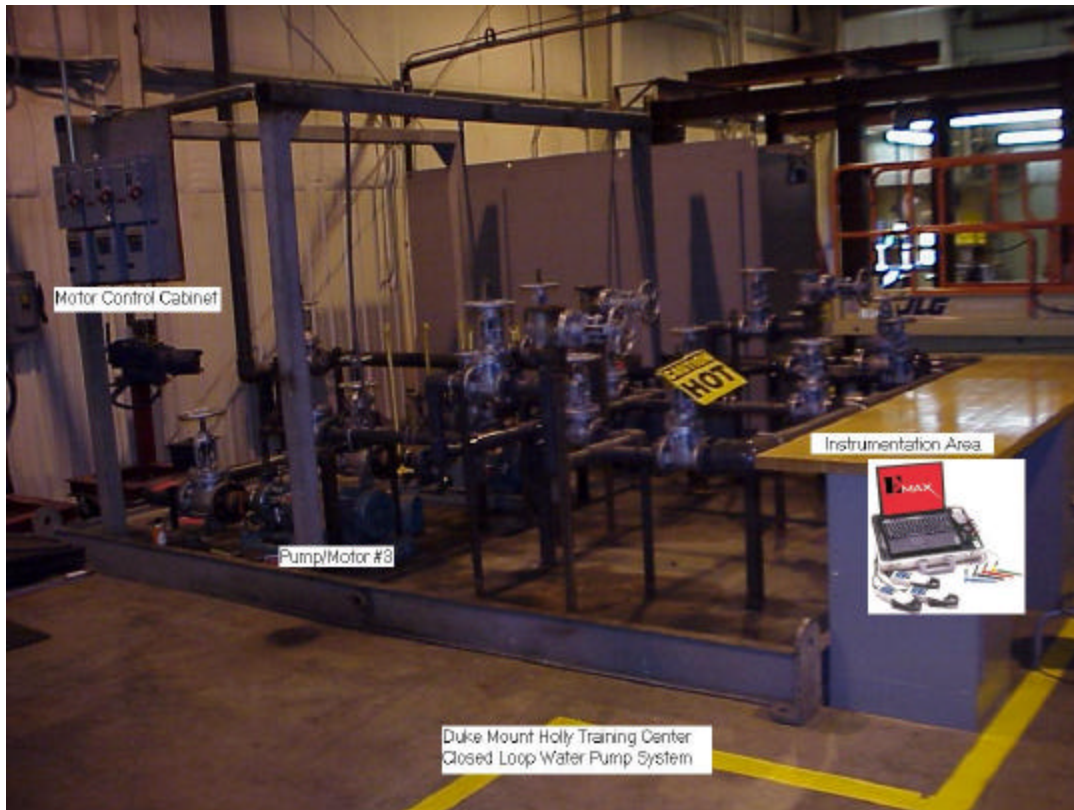
Figure A.1: Closed Loop Pumping System at Duke Mount Holly Training Center
