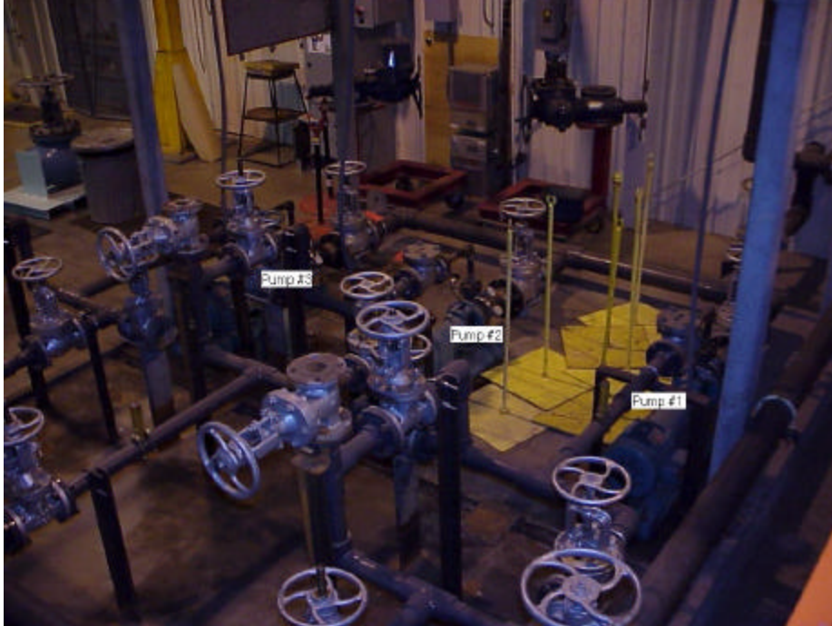
Figure A.2: Three Pumps in Parallel can be used in any combination
