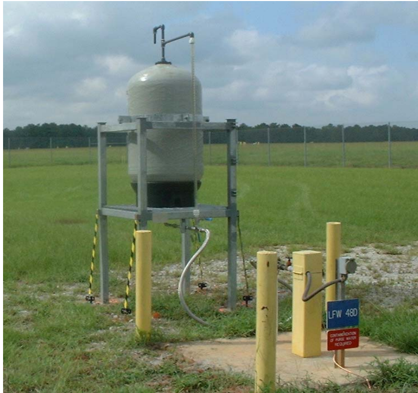
Figure 4. PWMS Tank Unit
