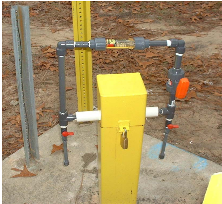
Figure 5. PWMS Tankless Unit Above-ground Portion
