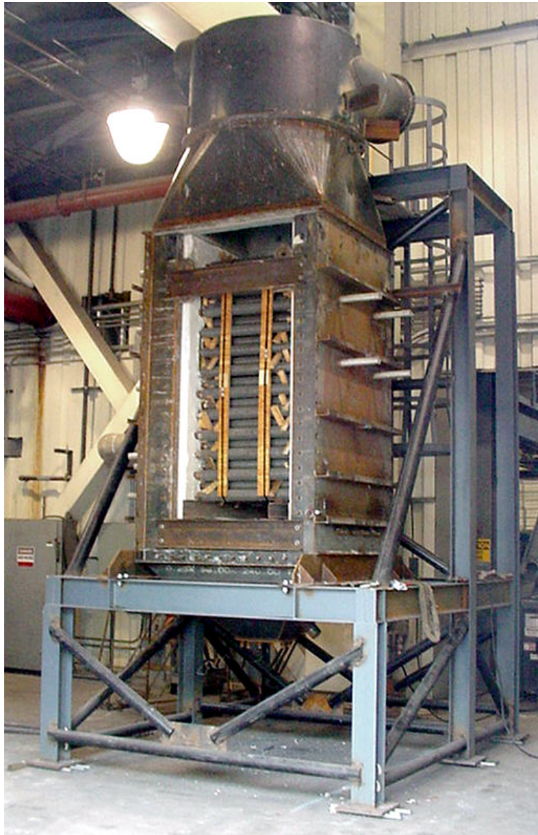
Figure 5.4-7: MBHE with Tube Bundles Installed
