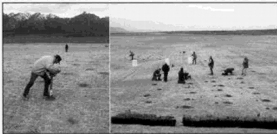
Figure 3-19. Digging holes with a power auger (left) allows the operator to provide sufficient holes and keep ahead of the planting crew (right).
