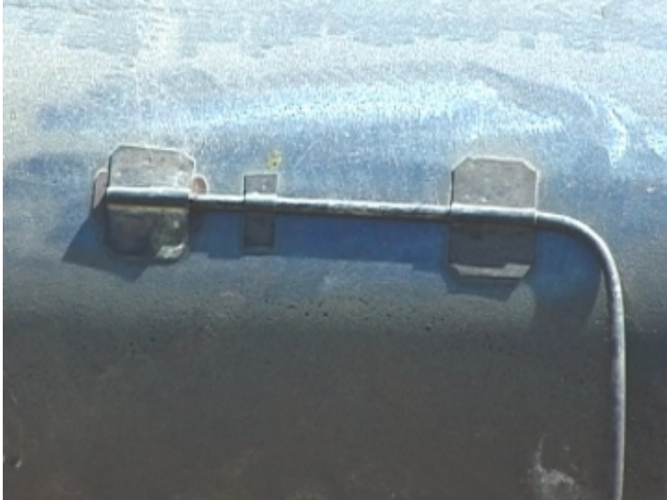
Figure A-2. Header Thermocouple Attachment
