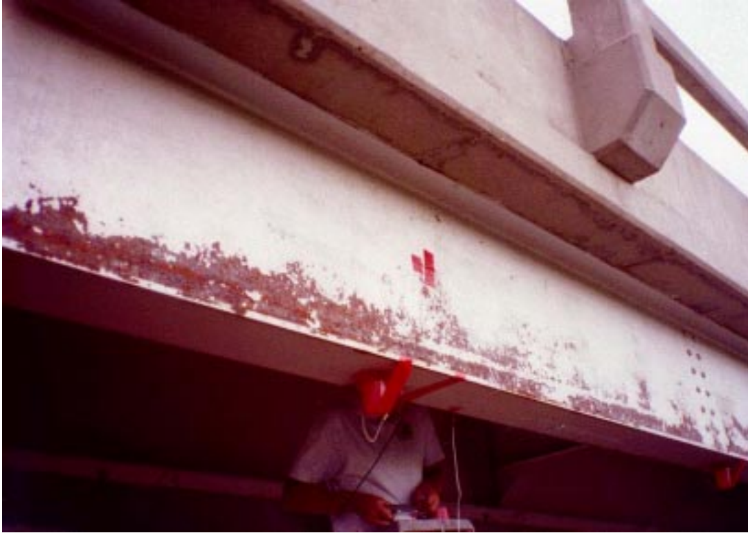
Figure 12. Deterioration of paint on west exterior girder.
