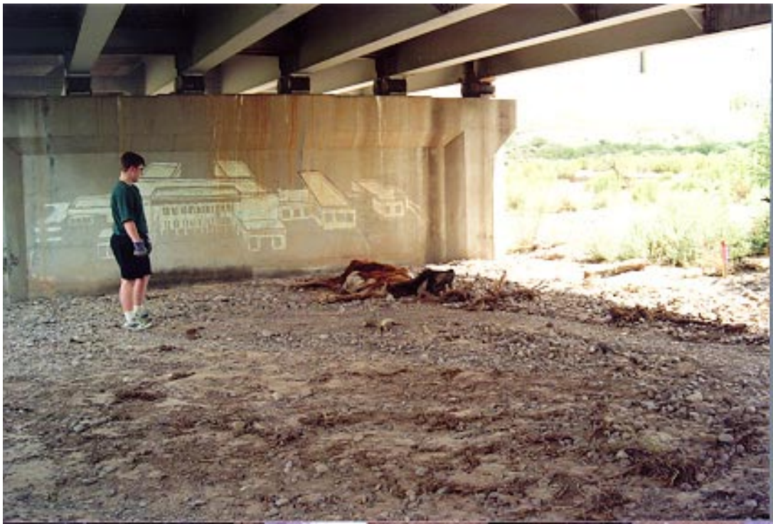
Figure 15. Dead cow located underneath an area of the bridge where instrumentation would be mounted.
