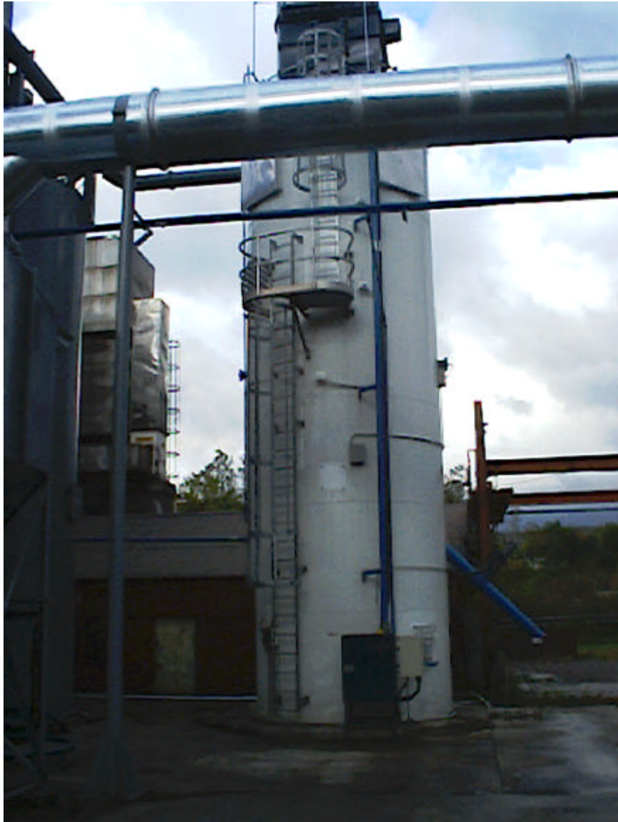
Figure 9 Char Storage Silo
