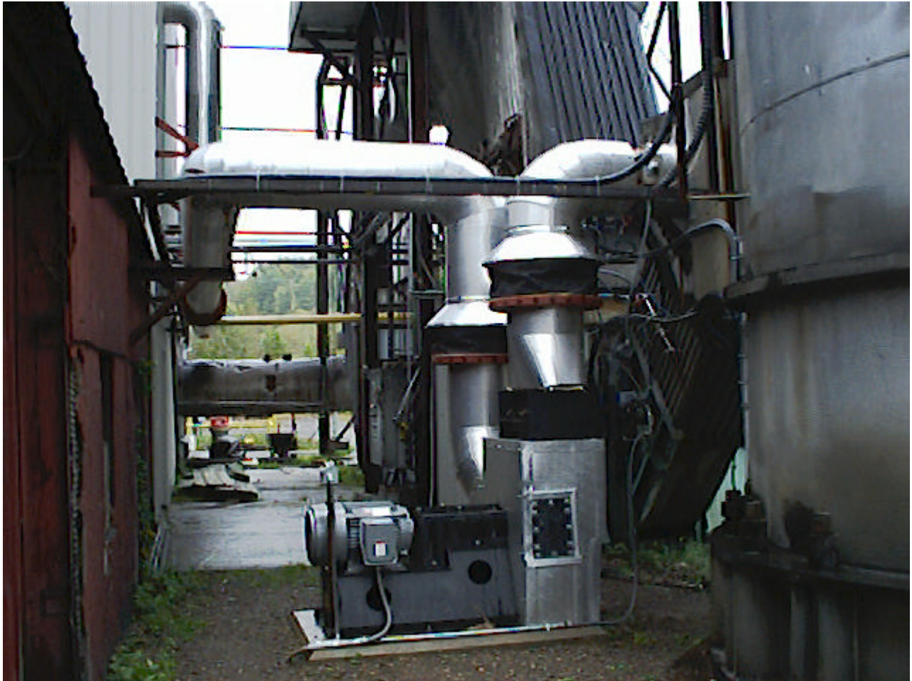
Figure 12 Flue Gas Recycle Piping
