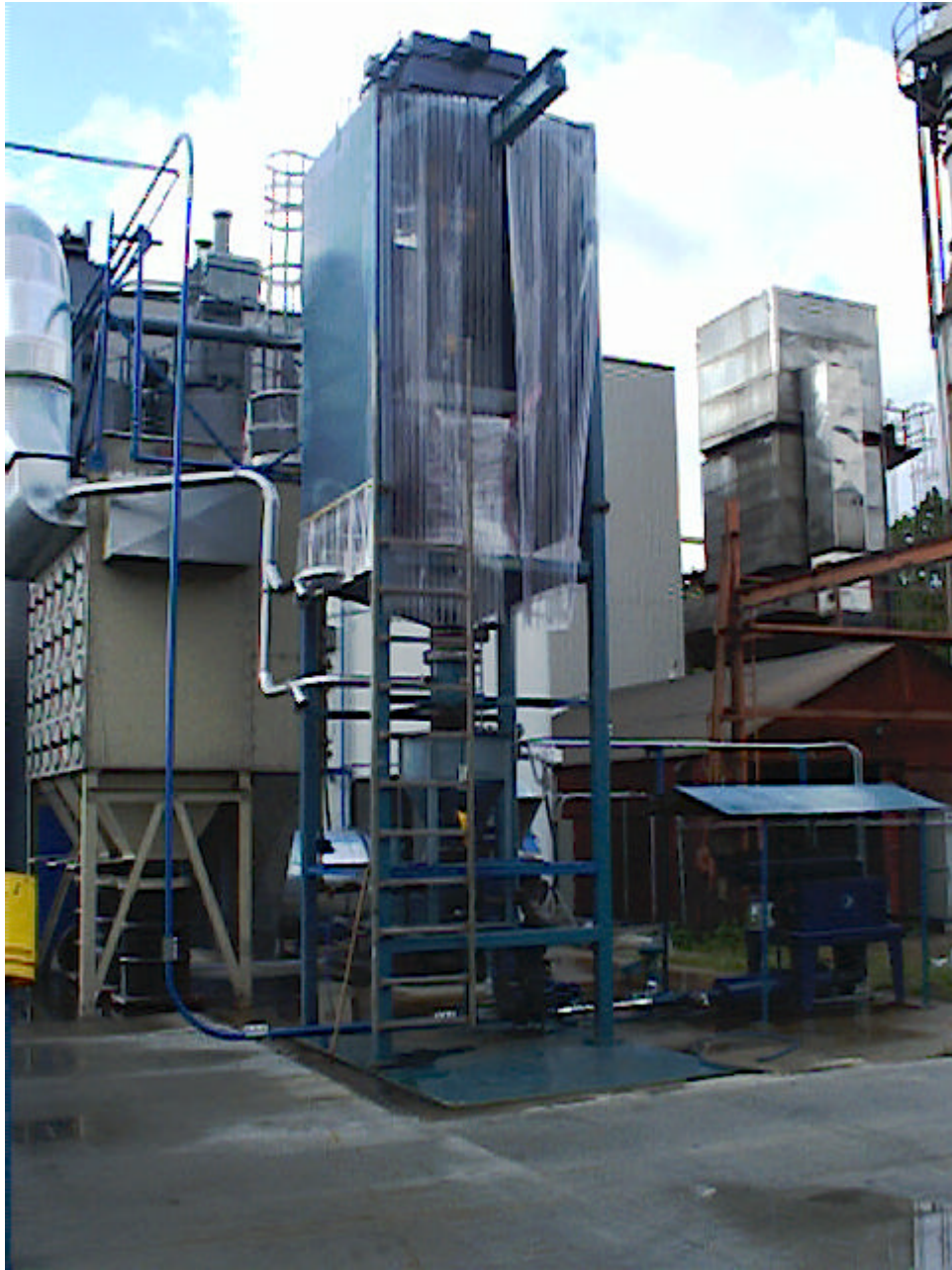
Figure 13 Pulverized Coal Unloading System
