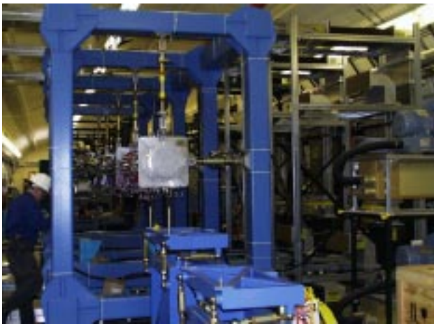
Fig. 3. LEDA RFQ installed in the beam tunnel.
