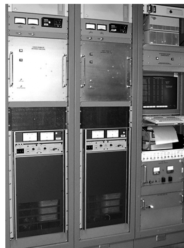
Figure 3. Two amplifiers (center of racks) and monitoring computer on right. DC power supplies are at lower left.
