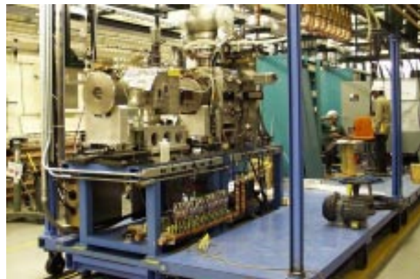
Fig. 2. LEDA injector installed in the beam tunnel.
