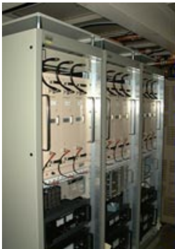
Figure 1: New rf system.
