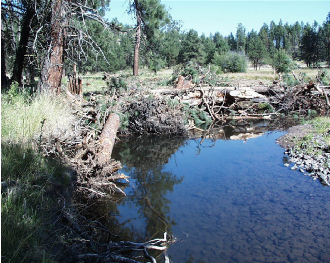
Figure 2. An engineered log jam (ELJ) constructed on Meadow Creek, Site 15, July 1999. Whole trees up to 30 inches in diameter and 80 feet in length were placed revetment style along an outside bend to stabilize the bank and enhance the quality of an existing pool. The largest tree had a 10 ft. diameter root wad that will provide hiding cover for juvenile steelhead. Tree tips were partially buried and placed outside of the bankful area to provide stability during winter flows and ice events.
