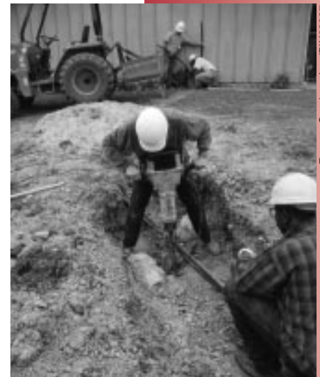
Workers drilling well outside of the base for the ground-source heat pump.
