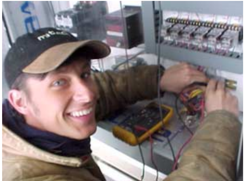
Figure 9. Troubleshooting controller components at Kotzebue
