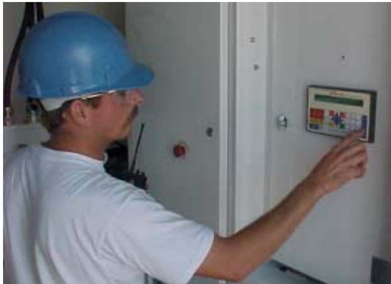
Figure 6. Zond technician adjusting controller setpoints
