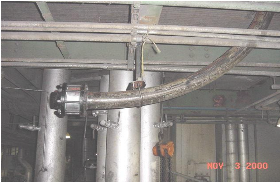
Figure 7. Piping at the Albright Generating Station
