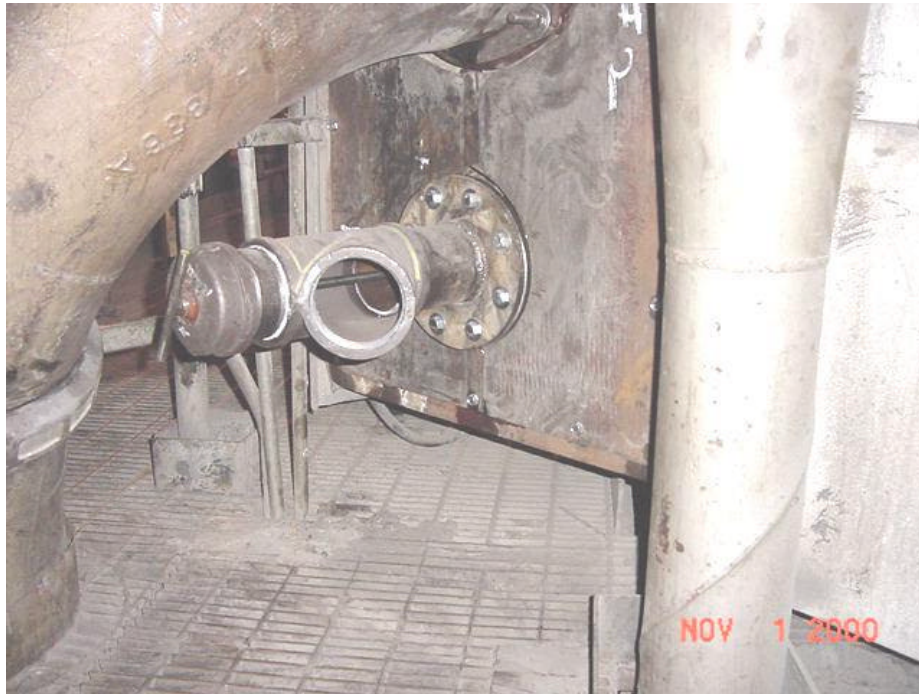
Figure 8. Piping Connections at the Albright Generating Station
