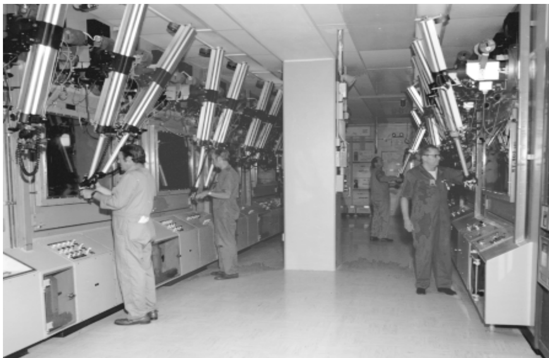
Figure 2. Plutonium Fuel Form Facility Hot Cell, Building 235-F
