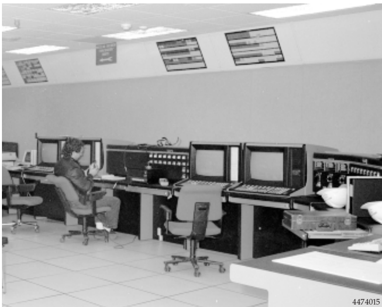
Figure 4. Modern control room for replacement precipitators
