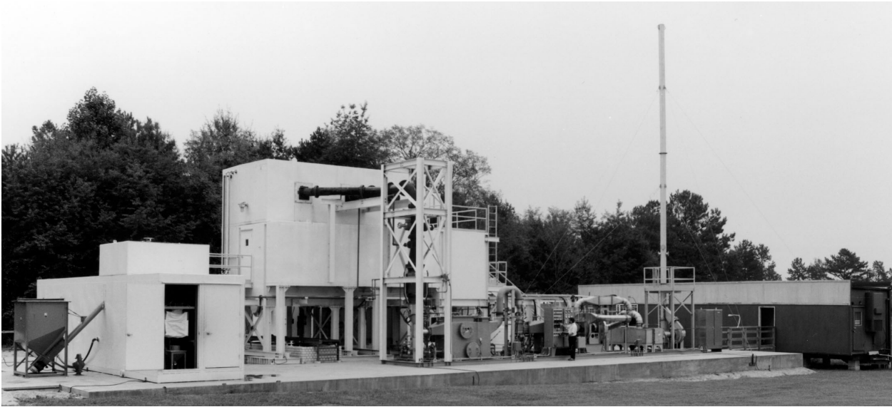
Figure 2. Transportable Vitrification System in the field. Composed of 5 modules, a feed batch preparation module (left) with an exterior waste tank or hopper, a melter module (center double story), an offgas module (along front face of concrete pad with a 40-foot tall offgas stack), a control/power supply module (behind the offgas and melter module). Co-designed by EnVitco Corporation and SRTC (U.S. Patent 5,611,766).
