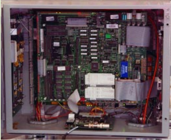
Figure 2. Argus field processors are microprocessor-based devices that verify badge information transmitted from remote access panels against locally stored encrypted access authorization databases.
