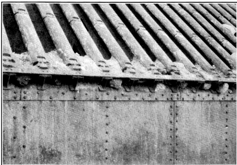
B. VIEW OF PART OF THE GRIZZLY SHOWN IN PLATE IX, A. THE OPENINGS BETWEEN THE STEEL BARS ARE ABOUT 8 INCHES WIDE.
