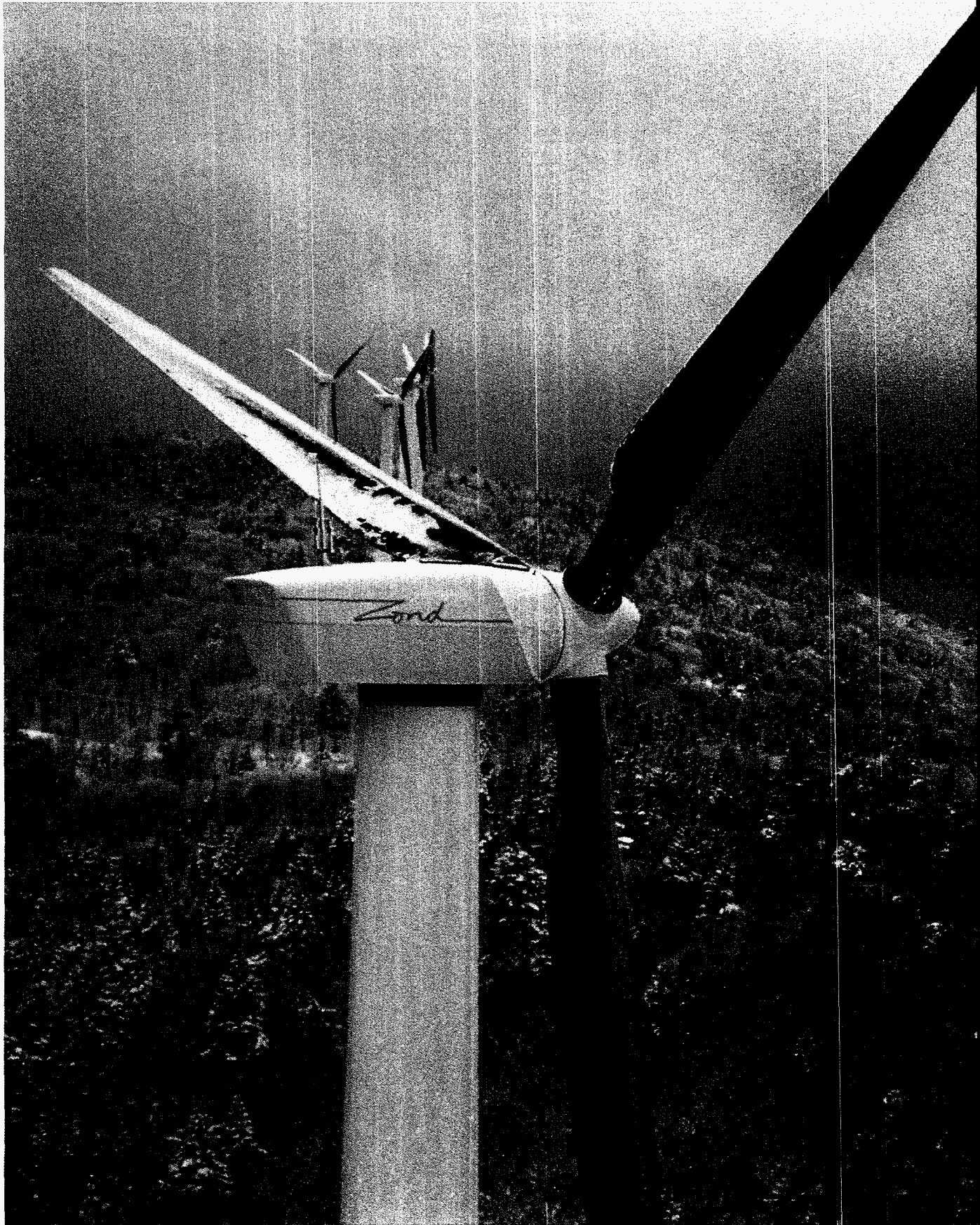
Construction crews cut as few trees as possible to build the Searsburg wind power plant. Now that construction is complete, the area around the tur
