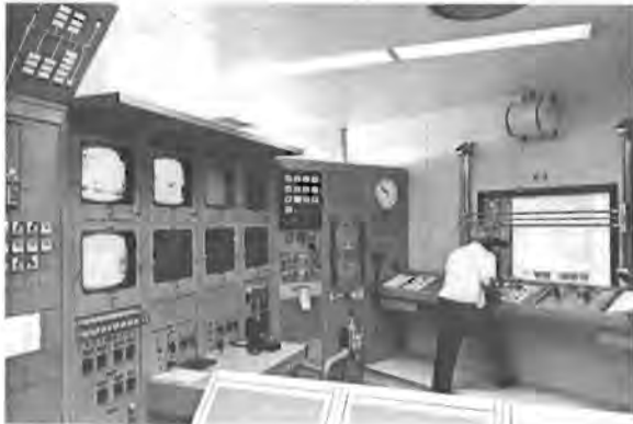
Figure A-8. Master Control Room
