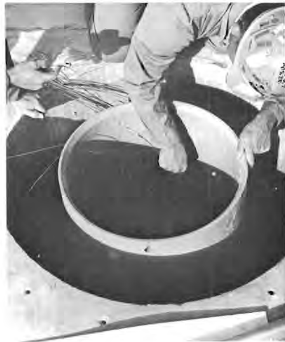
Figure B-59. Insertion of Thermocouples Into Drywell and Into Canister Through Shield Plug
