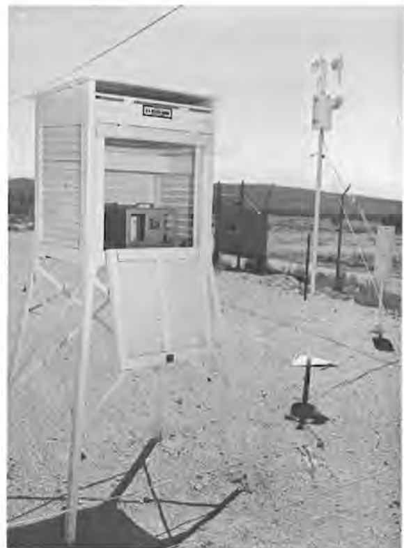
Figure A-26. E-MAD Weather Station
