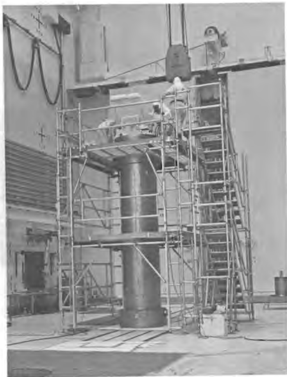
Figure B-26. Shipping Cask Positioned in Cask Work Platform
