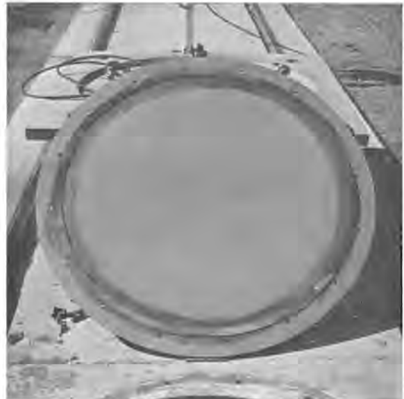
Figure 3.2-21. Drywell Cover Plate Showing Neoprene Gasket
