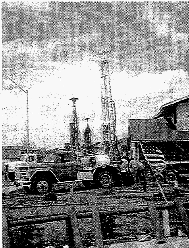
Fig. 1.4. A rig drilling vertical boreholes for the ground heat exchangers. A total of 1,834,652 ft of 4 1/8-in. vertical bore was drilled for the vertical borehole heat exchangers.
