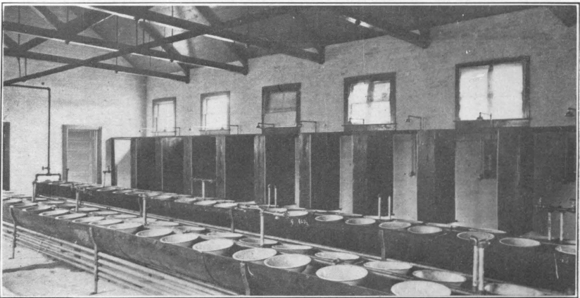
B. A SEMICIRCULAR WASH TROUGH WITH BASINS IN POSITION; HEATING PIPES UNDER THE TROUGH AND SHOWERS IN THE REAR.
