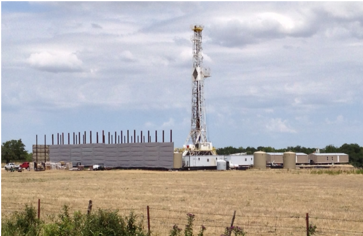
Fig. 3 Constructed drilling site in the study area with acoustical barriers and accessory structures
