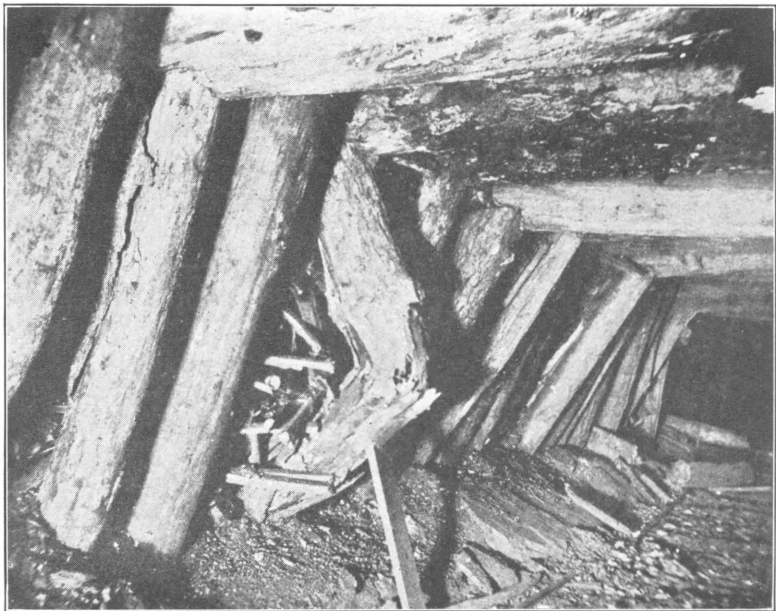
B. FAILURE OF AN UNTREATED LOBLOLLY PINE POST BY DECAY. DIRECTLY TO THE LEFT OF THE BROKEN POST IS A POST PLACED AT THE SAME TIME AND TREATED WITH ZINC CHLORIDE. AFTER U. S. FOREST SERVICE.
