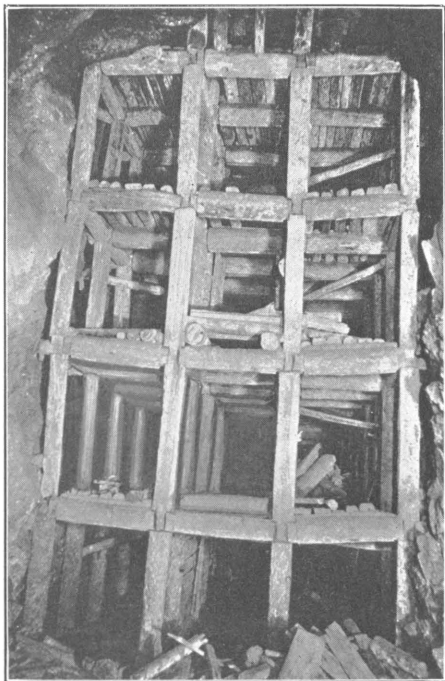
1. BUTTED-POST METHOD OF FRAMING SQUARE SETS. NOTE ABSENCE OF BLOCKING BETWEEN THE ENDS OF THE TIMBERS AND THE WALLS.
