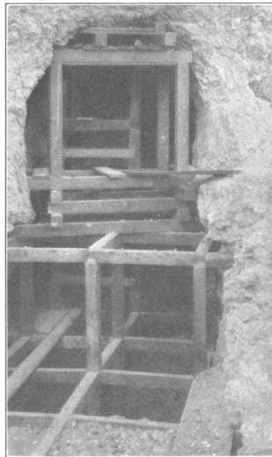
2. BUTTED-CAP METHOD OF FRAMING SQUARE SETS. NOTE HOW THE LONG STRINGERS ARE PLACED OVER THE JOINT OF THE TIMBER SET.
