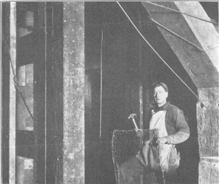
B. METHOD OF PLACING METAL LATHING ON SHAFT TIMBERS BEFORE APPLYING GUNITE.
