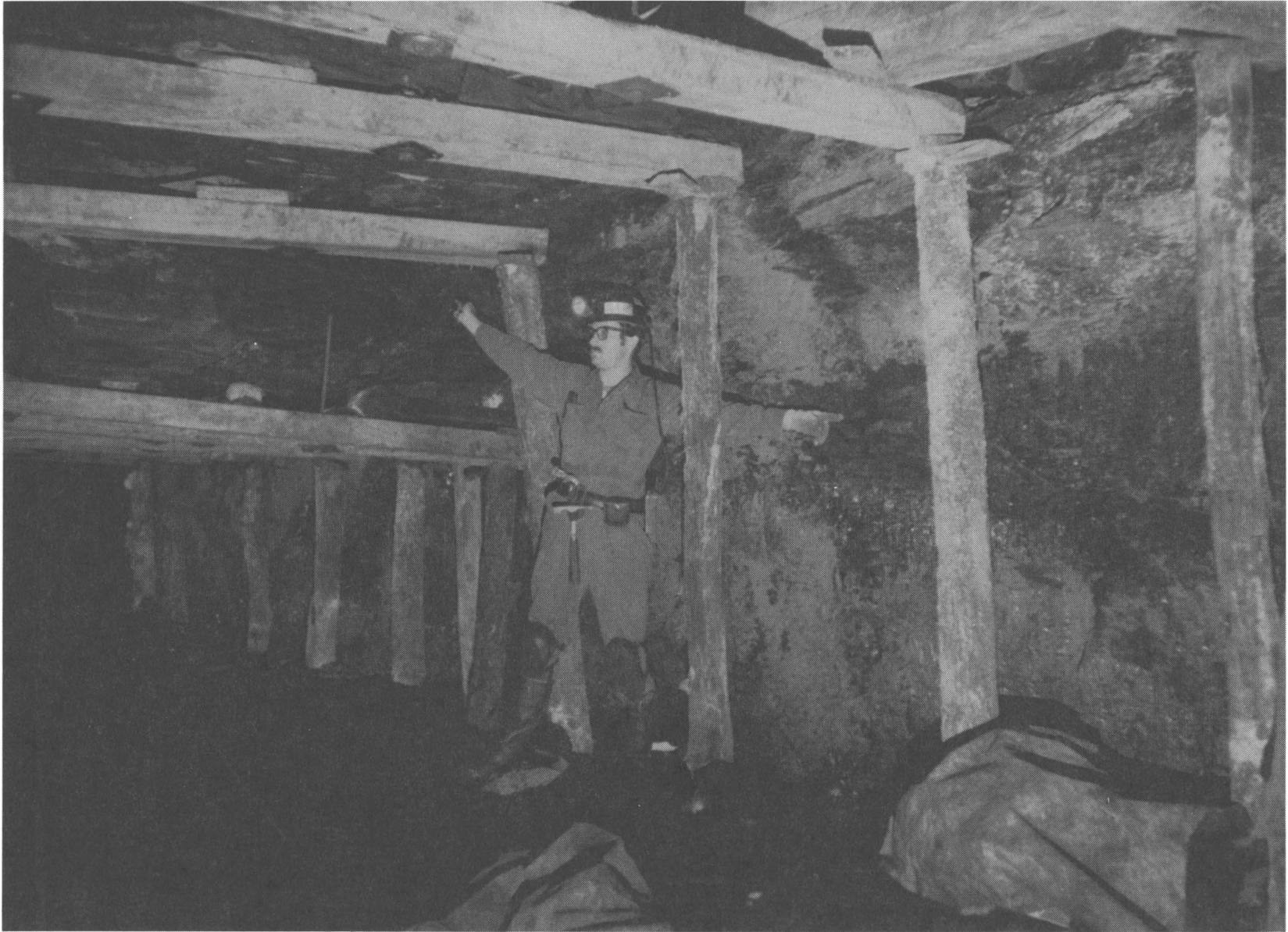
FIGURE 17. - Photograph of thrust fault and associated roof fall within shale roof-rock of the main entries.
