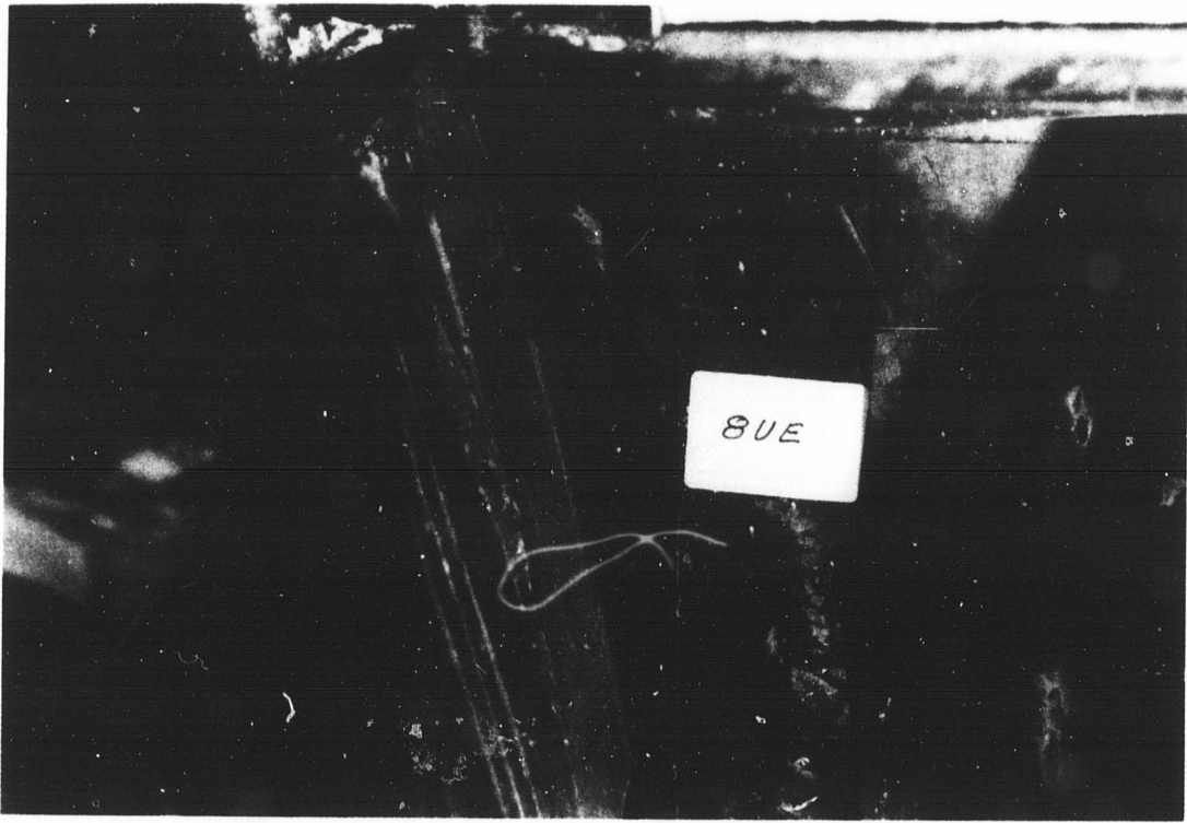
Figure 5.23 Tearing of top end of north clip angle at location 8UE.
