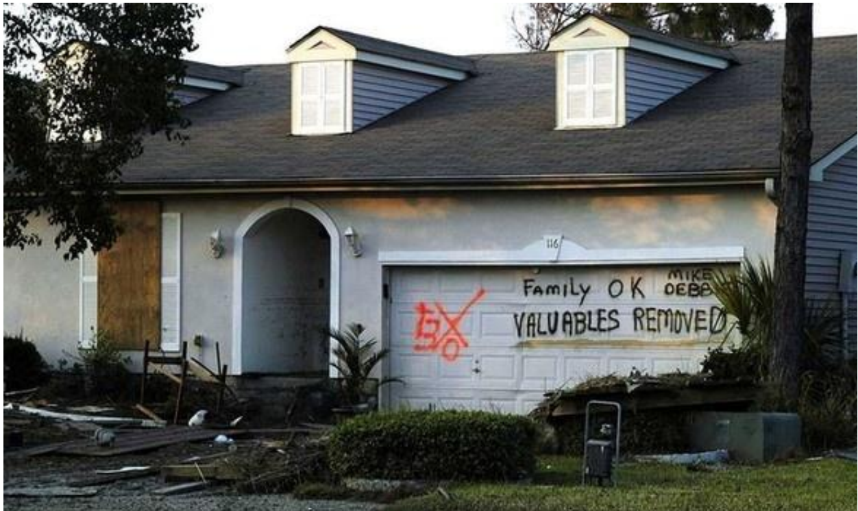
Figure 41. Residents of this south Slidell home spray-painted a message on their garage door that assured friends and family they were safe. The message that they had removed valuables from their home may have been for family or potential looters. Photo taken by Tisha Slagle, September 19, 2005.
